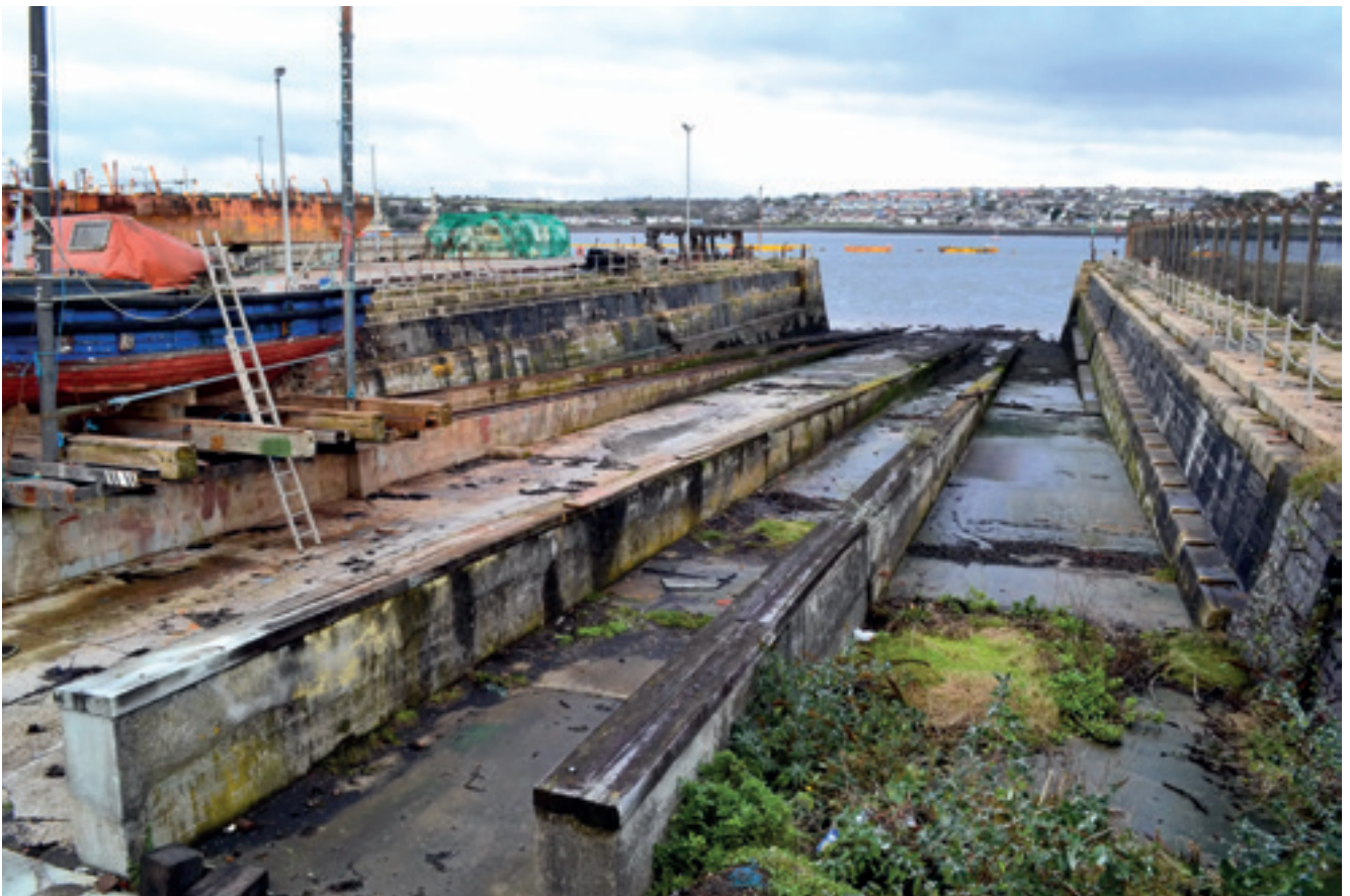
Historic structures such as this slipway at Pembroke Dock – which was second only to Plymouth for building Royal Navy ships in the mid-late C19th – may be capable of sensitive reuse in supporting the wave and tidal energy sector. Image © Antony Firth/Fjords.
