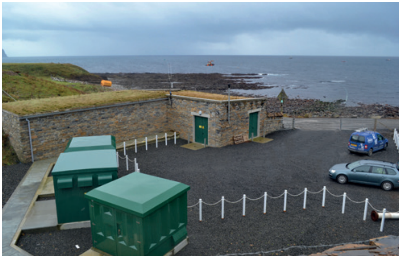
Onshore facilities at the EMEC test site at Billia Croo, Orkney, with the test site itself in the background. Image © Antony Firth/Fjodr.
