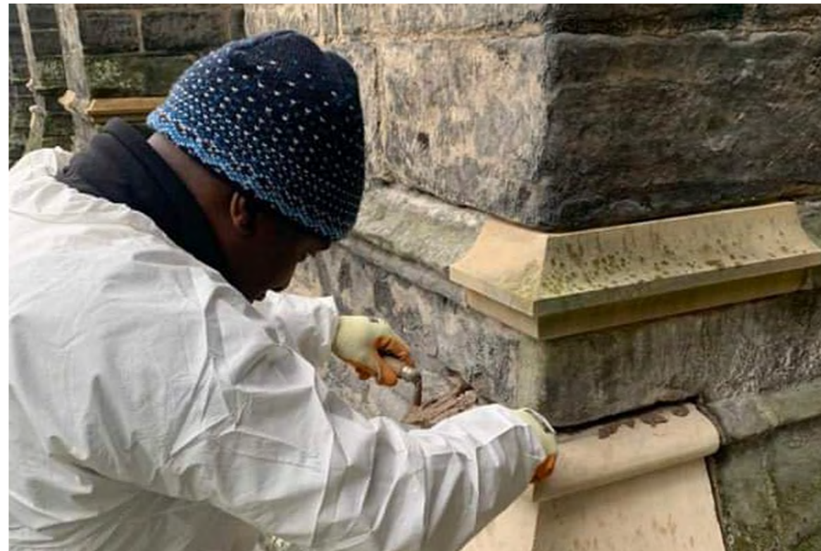
The skilled work of HES masons and grounds team is integral to the protection of Scotland's historic assets and could be at the forefront of HES' public facing offer.
