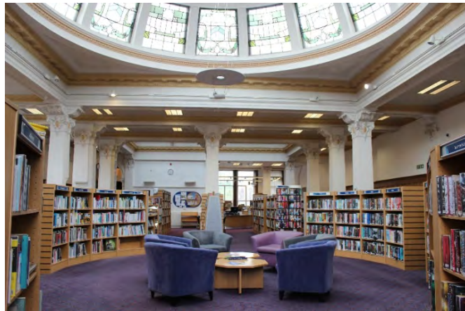
Figure 40: Glazed dome over the former reading room at Rutherglen Library. This is one of the best-preserved glazed domes in Scotland © South Lanarkshire Libraries
