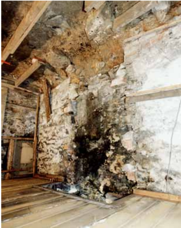
Illus. 11 The W gable wall showing an area of exposed wall core is formed of orange subsoil and has been raked out and replaced with brickwork wherever it remained exposed (Historic Scotland)
