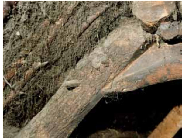
Illus. 19 Details of pegging on the E face of the E cuppill (Historic Scotland)
