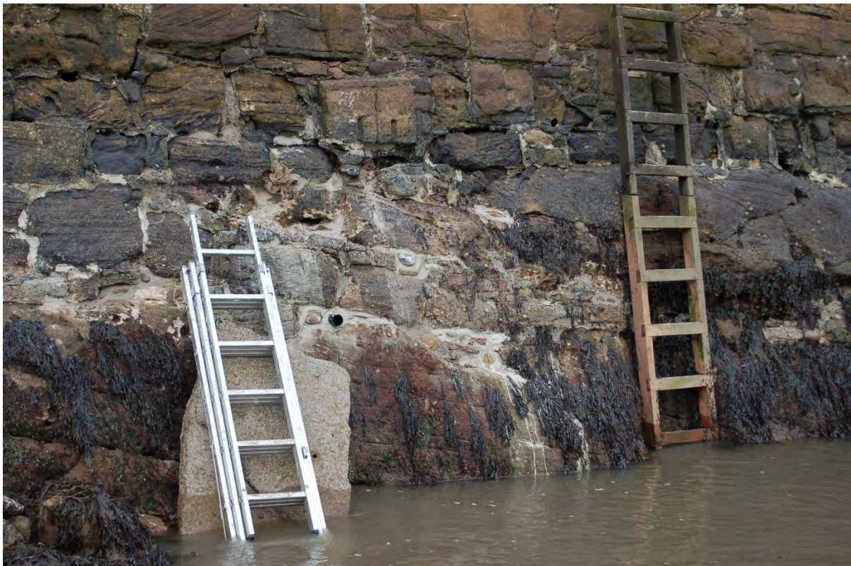
Figure 8. Partially completed pointing of the face of the main pier to the grouting trial.
