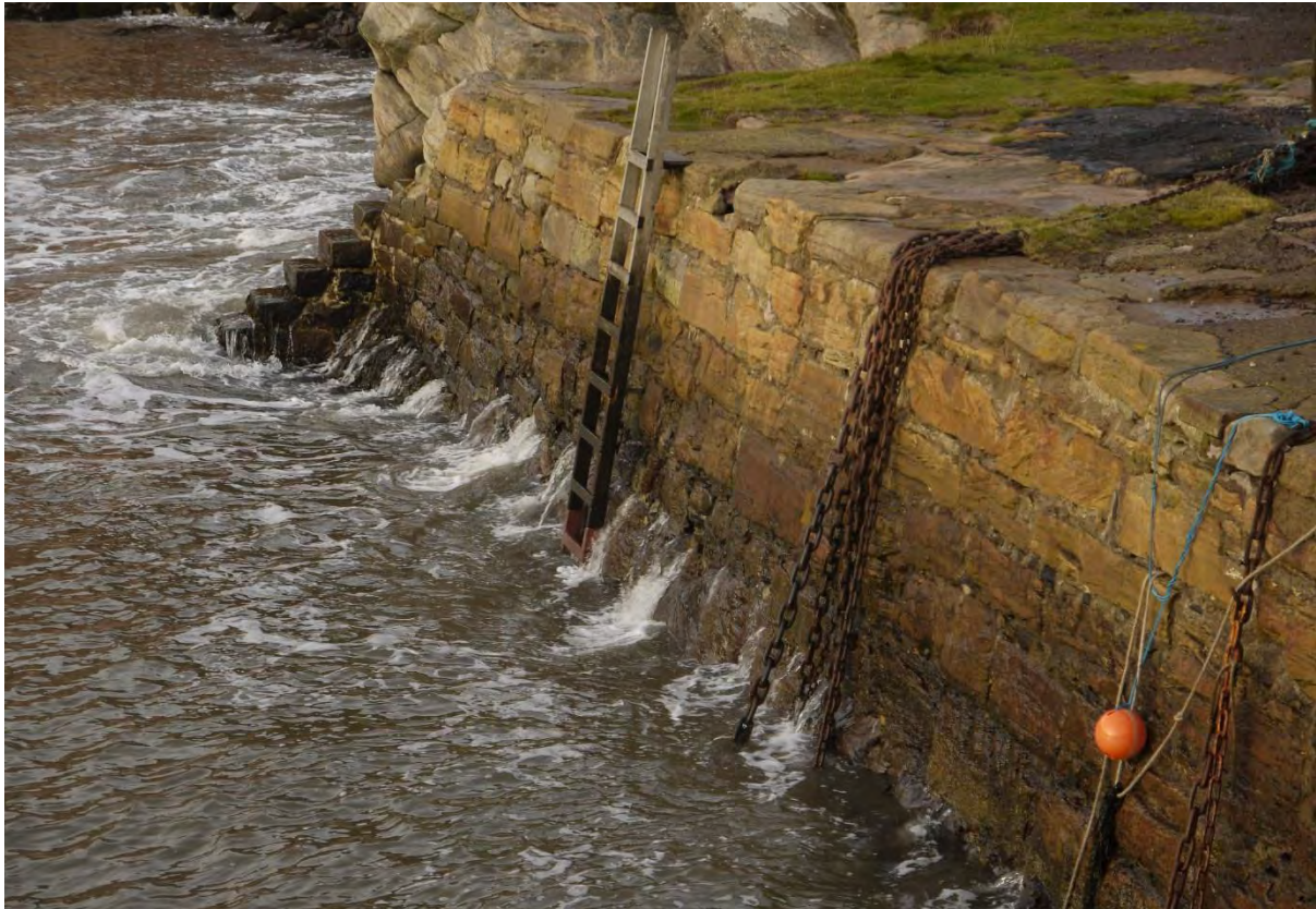
Figure 4. Receding wave action revealing the presence of water in the voids of the Main Pier. The trial works were carried out in this area of the harbour.
