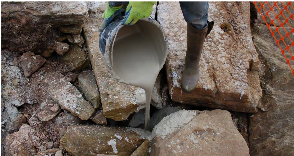
Figure 11. Pouring in the grout into the opened core with a builder's bucket.
