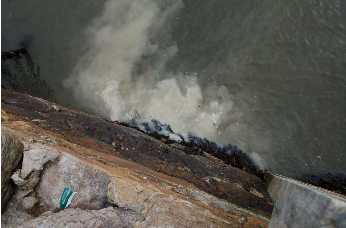
Figure 12. The grout was able to flow some distance within the structure and can be seen coming out of the pier face approximately 10 metres from the point of pouring.
