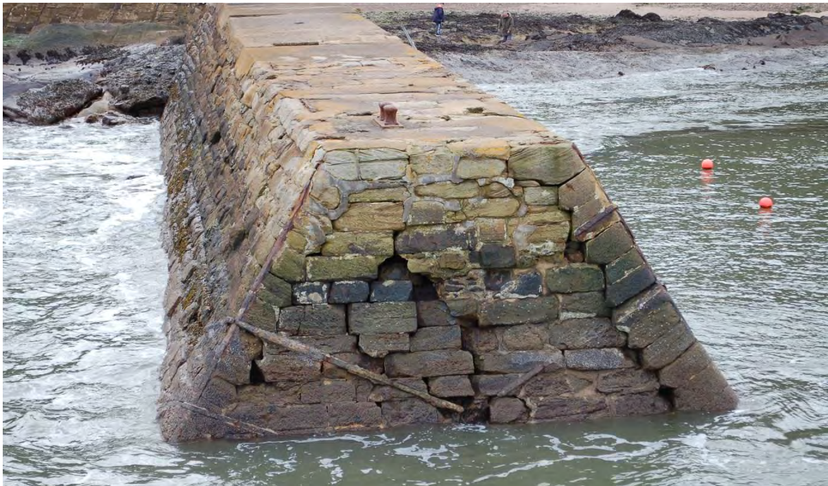
Figure 3. Masonry movement due to loss of core material can be clearly seen in this image of the north end of the Boyne Pier.
