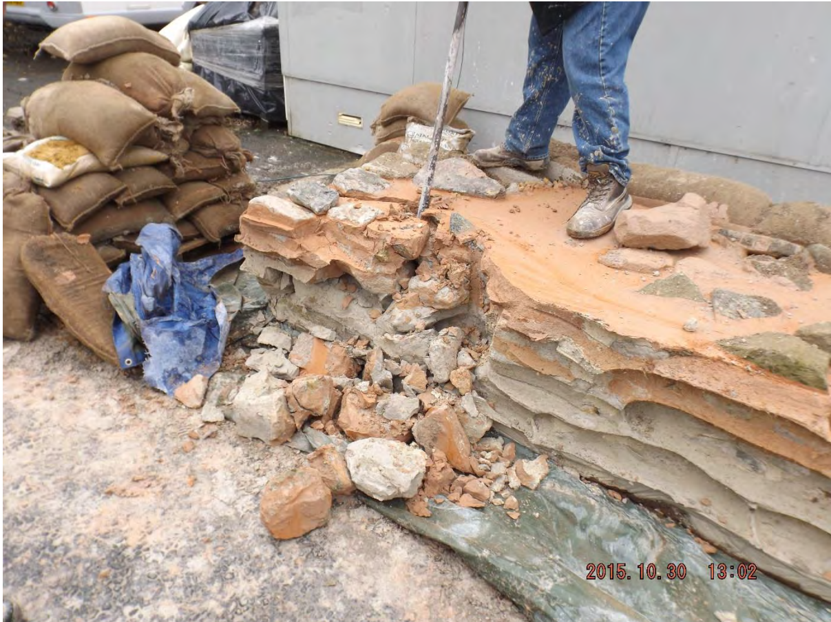
Figure 7. Opening up the grouting rig to assess penetration and the degree of set of the grout.
