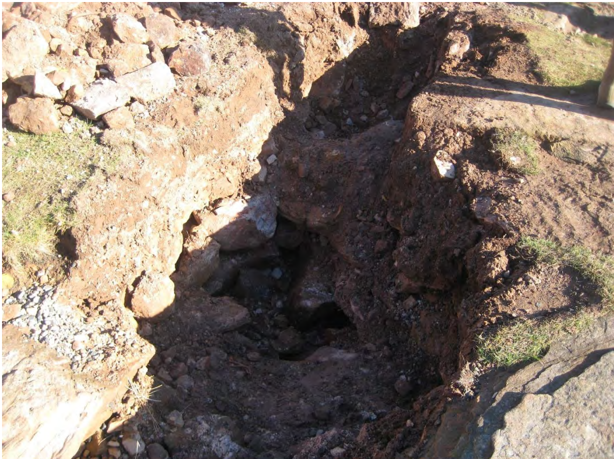
Figure 9. One of the pits opened up in the pier deck to expose the core beneath.
