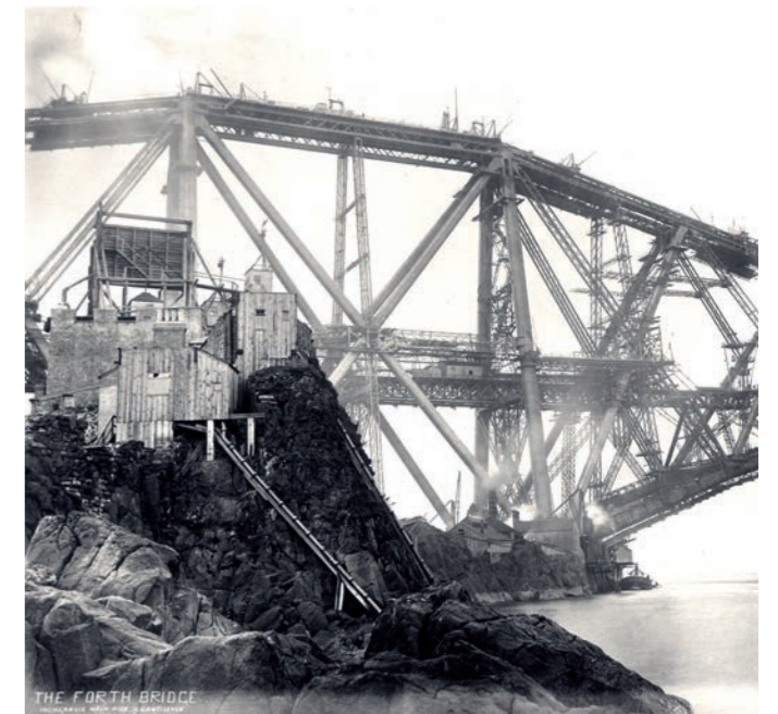
Inchgarvie north cantilever under construction in 1888. © Crown Copyright National Records of Scotland, BR/FOR/4/34/436.
