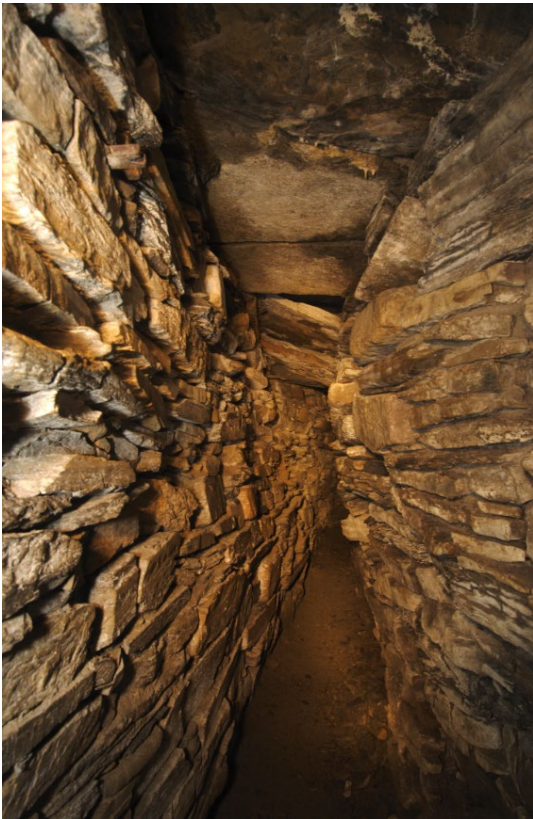
Midhowe Broch ground level gallery showing displaced lower courses and stone packing of gallery
