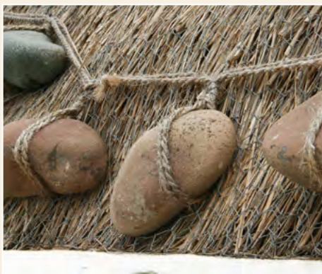
Fig 15. Weights and fixings should be regularly checked and secured.
