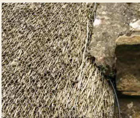
Fig. 10 Thatch with cement skew fillet, Fife.
