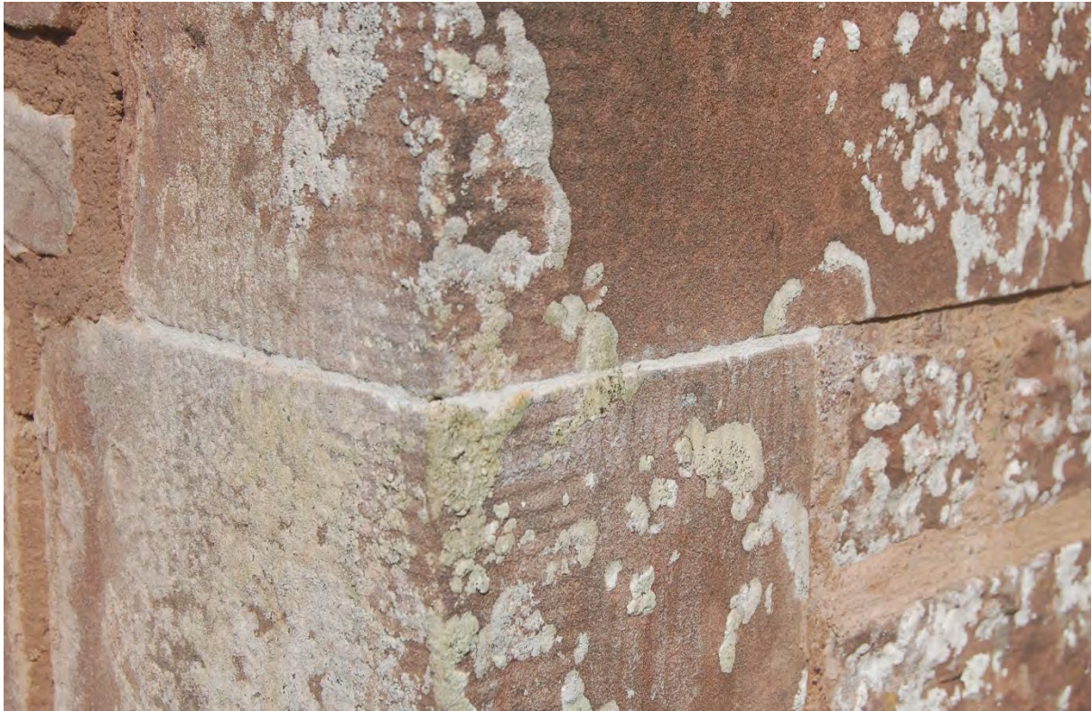
Figure 9. New ashlar pointing work on the narrow joints of the vestry gable quoins.
