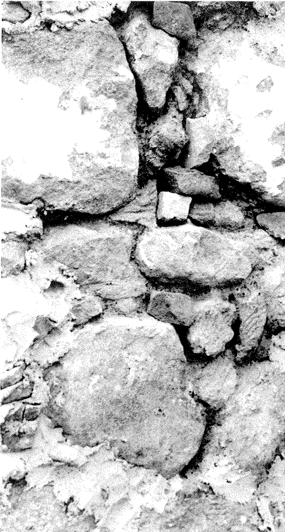
Fig. 38 Pinnings placed into joints. Note how stones generally make contact with each other.
