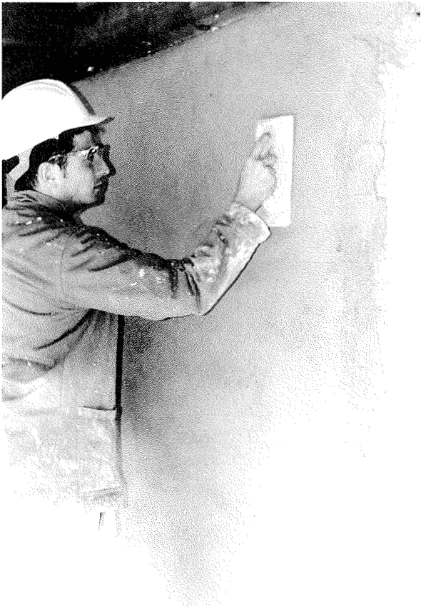
Fig. 90 Scouring (floating) in the second coat.
