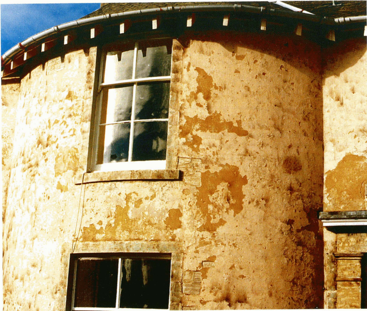
Fig. 21 Damage following removal of modern paint coating.
