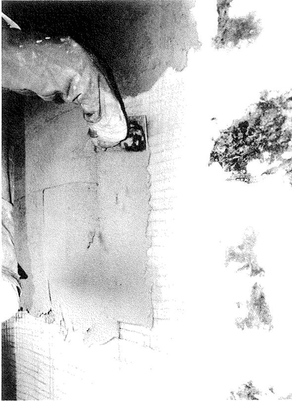
Fig. 88 Laying on a second coat. Note the amount of pressure being applied.
