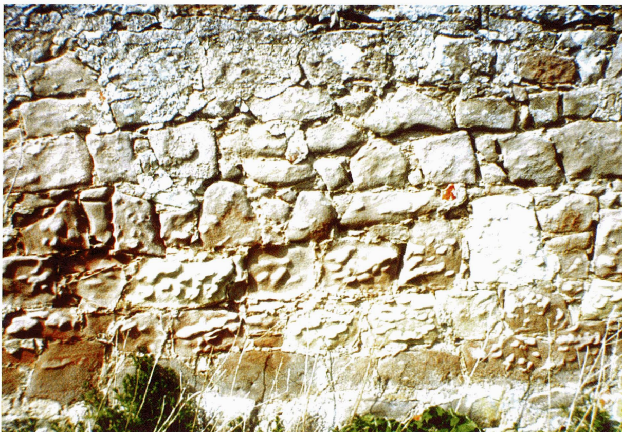
Fig.35 Heavily eroded masonry will require repair before harling.
