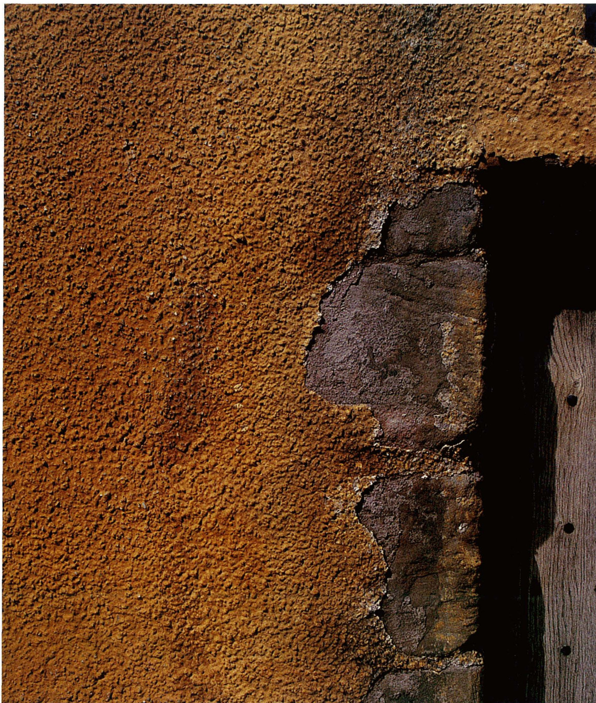
Fig. 15 Traditional lime harling subject to salt attack on badly contaminated masonry.
