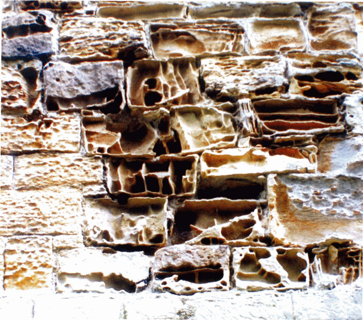
Fig. 40 Ashlar masonry suffering from deep erosion.
