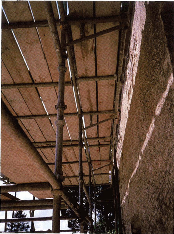
Fig. 57 Scaffolding with correctly placed uprights and removable inner boards.
