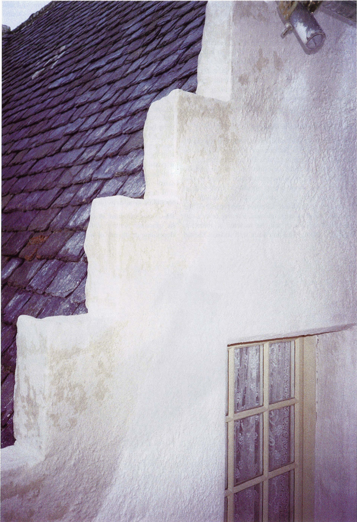
Fig. 53 Additional attention will be required to maintenance at vulnerable details such as harled crowsteps.
