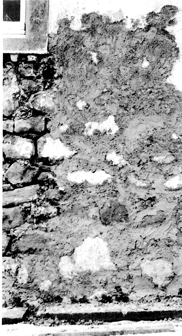
Fig. 39 Mortar filling out areas of shallow erosion in stones, ready for harling.
