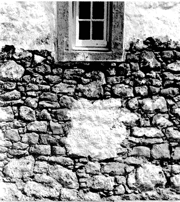
Fig. 62 Wall following removal of defective harling.
