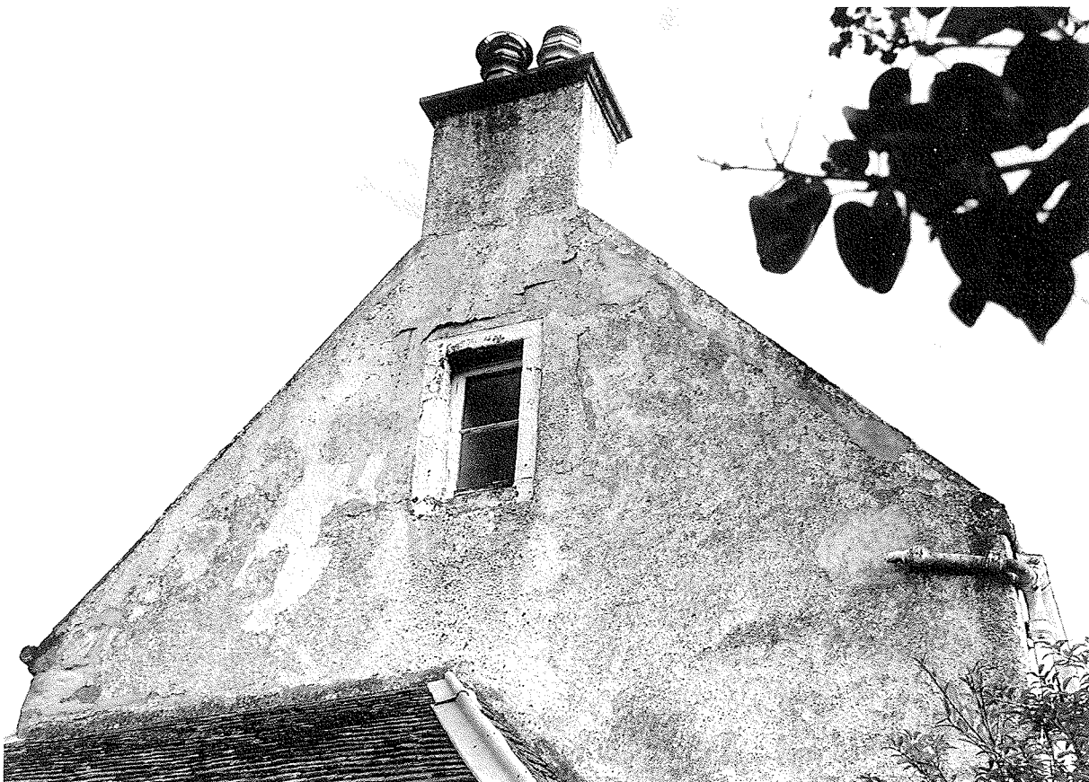
Fig. 52 Identify problem areas such as at chimneys, wallheads, below skewes and window cills.
