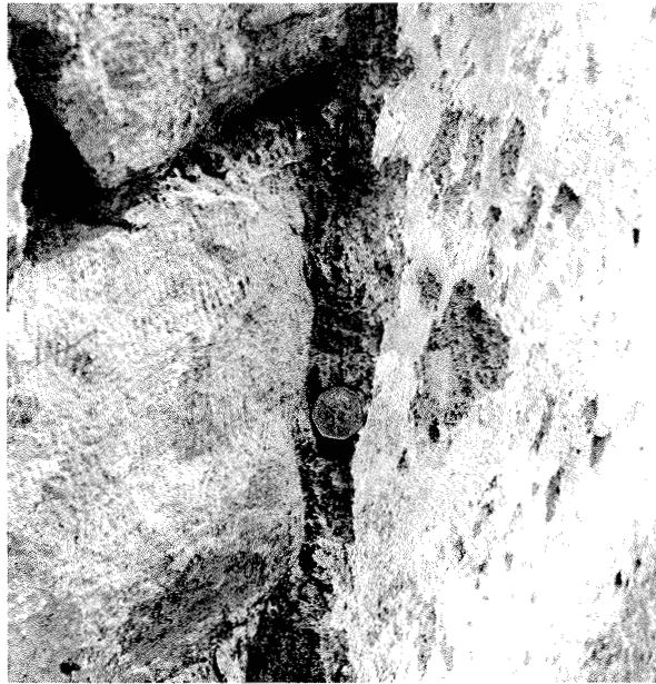
Fig. 61 Thickness of inappropriate former repairs to harling.
