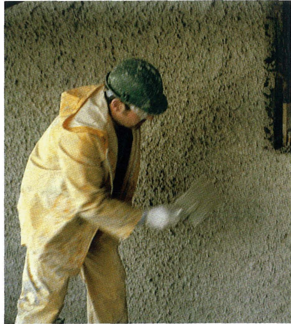
Fig. 26 Standing at right angles to the wall, harling is applied with a flick of the wrist. Care should be taken to avoid 'fan' patterns in the finished work unless to match the existing adjacent finish.
