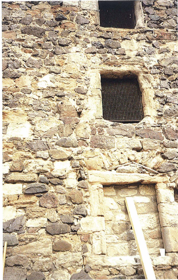
Fig. 23 Where masonry is eroded or pinning stones have been lost, surfaces require repair before application of harling or render.
