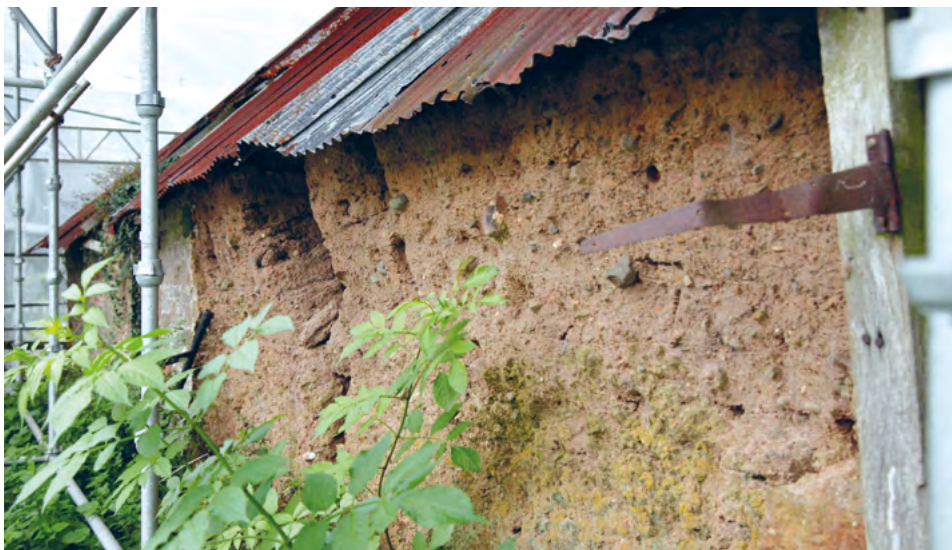
Fig. 4 Earth construction revealed following loss of the cement render.
