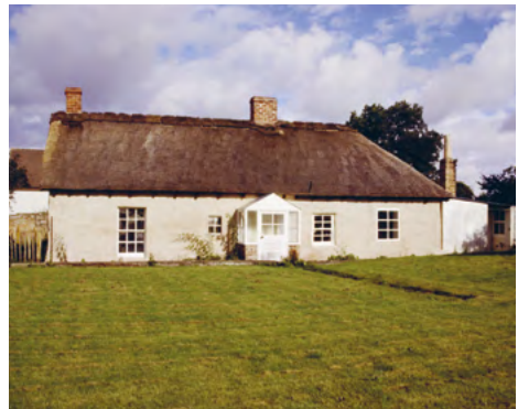
Fig. 6 This clay building has been lime harled to protect against the weather.
