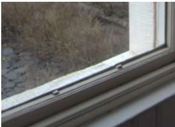
Fig. 14: Stumps of removed astragals showing the original 6 over 6 glazing arrangement.
