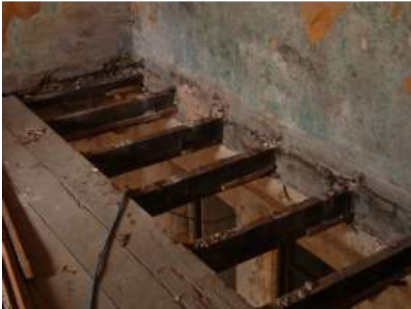
Fig. 17: Undersized timber floor joists resulting in movement across the floors.
