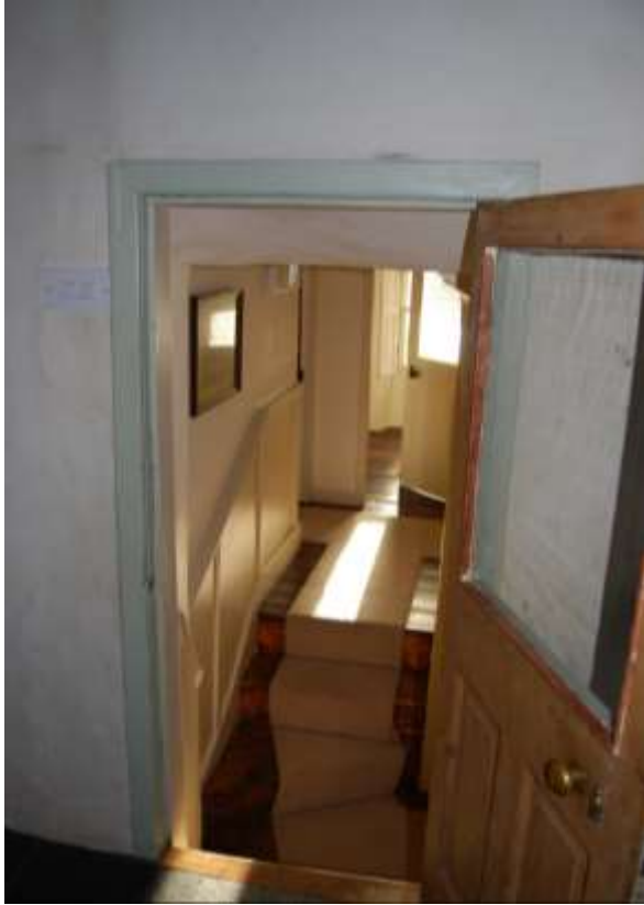
Fig. 6: Previous works creating a door opening from former stair window, allowing access to the later lean-to extension.
