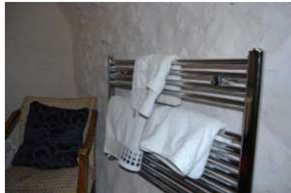
Fig. 34: Electric heating towel rails installed in the bathrooms for additional heat
