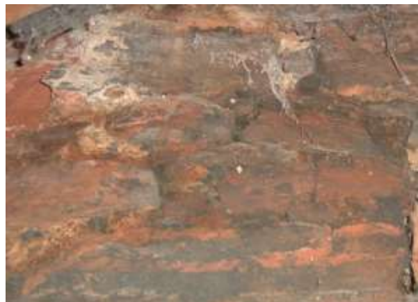
Fig. 5: Stained masonry and stone decay in the attic below chimney due to defective work above.
