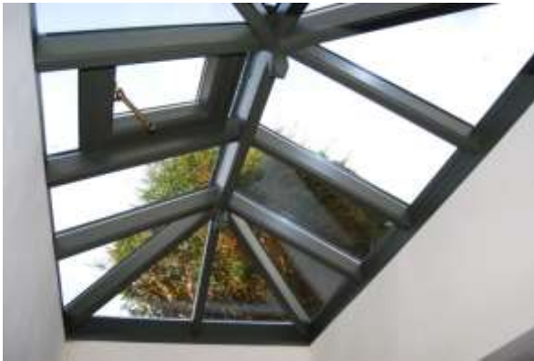
Fig. 7: Former lean-to roof, raised, thus creating extra space - now the current kitchen with large lantern light.
