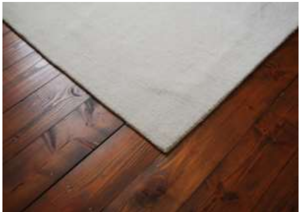
Fig. 20: New floor boards made by local sawmill, maintaining the width of the original boards.
