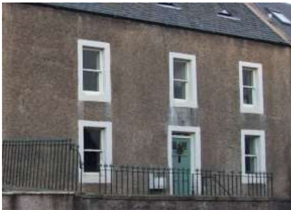
Fig. 12: Existing modern cement render.
