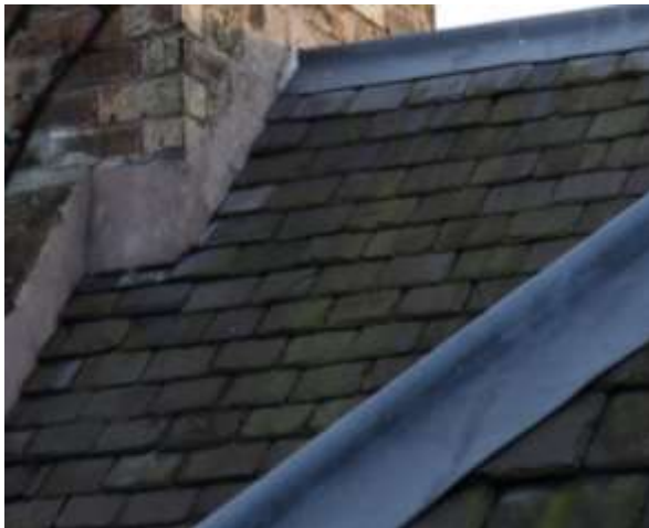
Fig. 11: Re-dressed, reinstated Welsh slate on the back pitch of the terrace, with replacement lead flashing.
