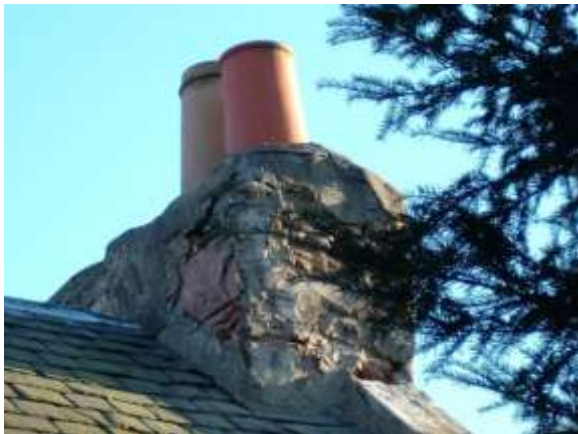
Fig. 4: The west chimney prior to works; note the lack of a cope and poor pointing.
