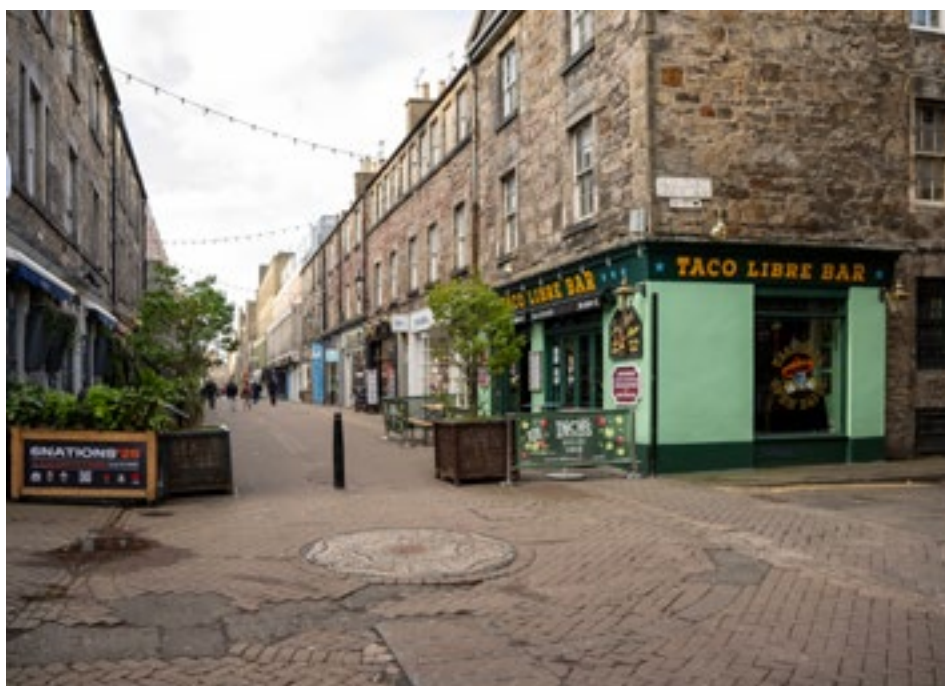
The Rose Street public realm in poor repair (© Neil Hanna)
