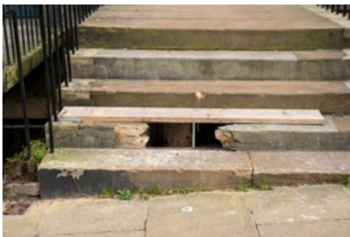
Howe Street step broken by falling masonry from Storm Eowyn (© Neil Hanna)
