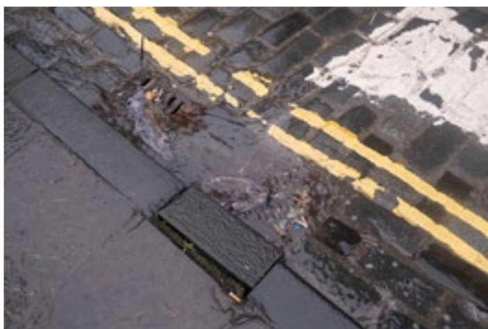
A clogged gutter drain (© Robin Mair Photography)
