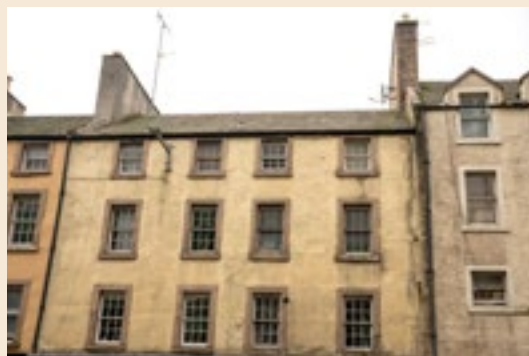
Poorly maintained traditional building surface in the South side of Edinburgh (© Neil Hanna)
