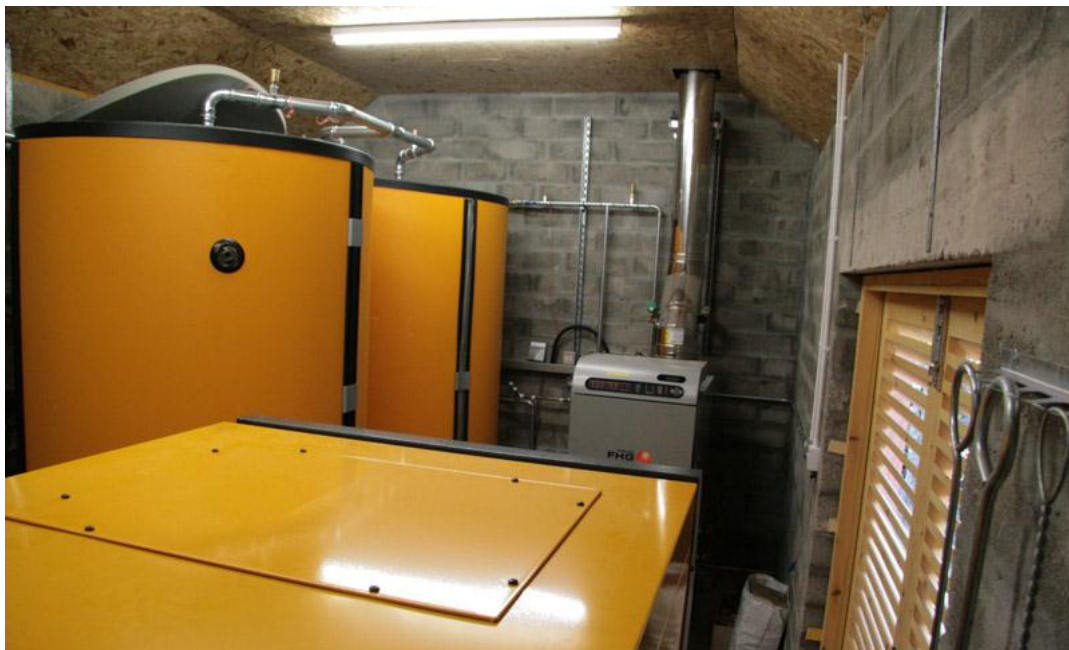
Fig 9: Looking across the large ETA Boiler toward the twin buffer tanks. To the right at the rear is the 20kW Fröling Log boiler. Photo taken before pipework insulated.
