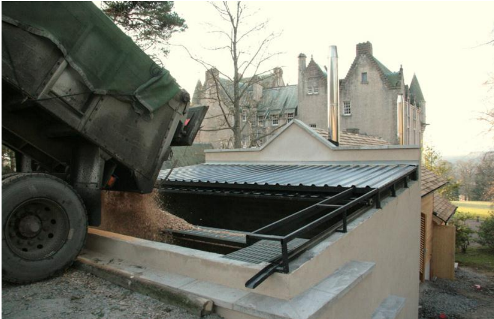
Fig 8: Wood chip (approx 20-22 cu.m.) brought from storage facility to the new boiler house. Photo taken before roof structure completed.
