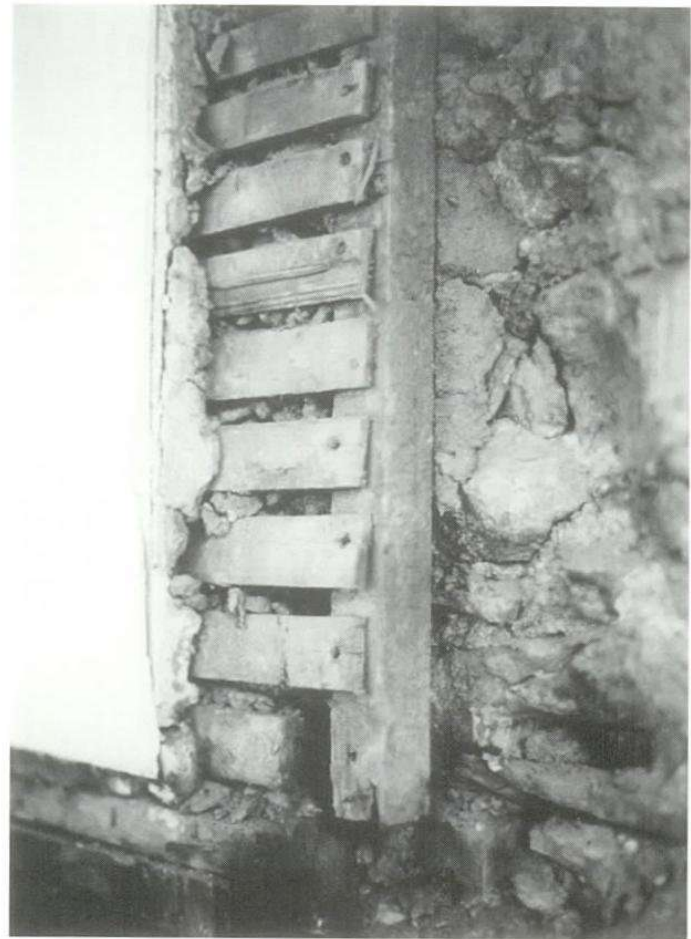
Fig. 7 Lath and plaster. To protect the plaster finish and supporting timbers from coming into direct contact with the more moist structural masonry-work, air spaces usually exist between the two. Whilst required to ensure effective environmental conditions, these spaces can also aid undetected fire spread.
