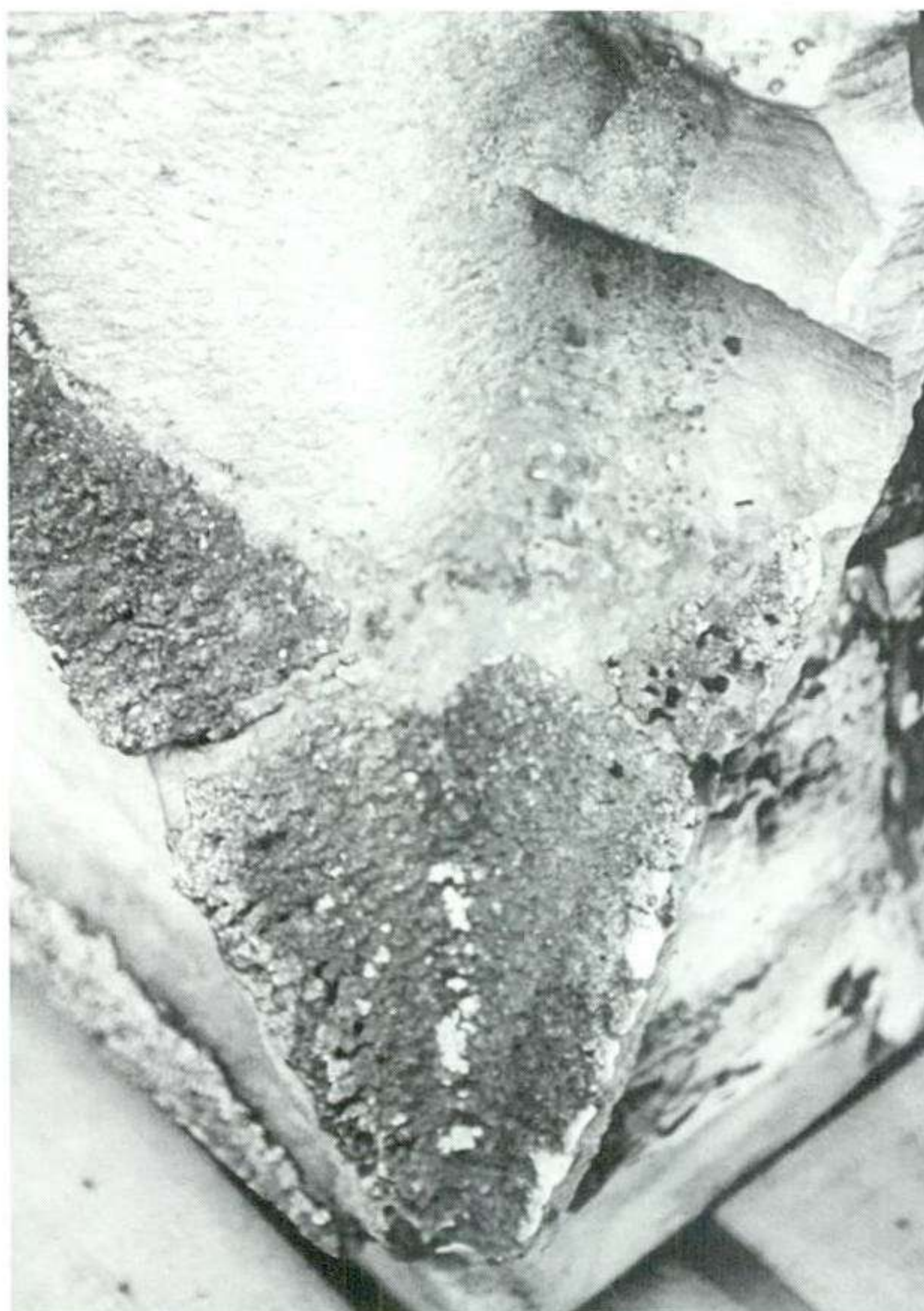
Fig. 1 Elgin Cathedral. Molten lead from the roof can still be seen bonded to the upper level masonry, resulting from torching of the Cathedral in 1390.
