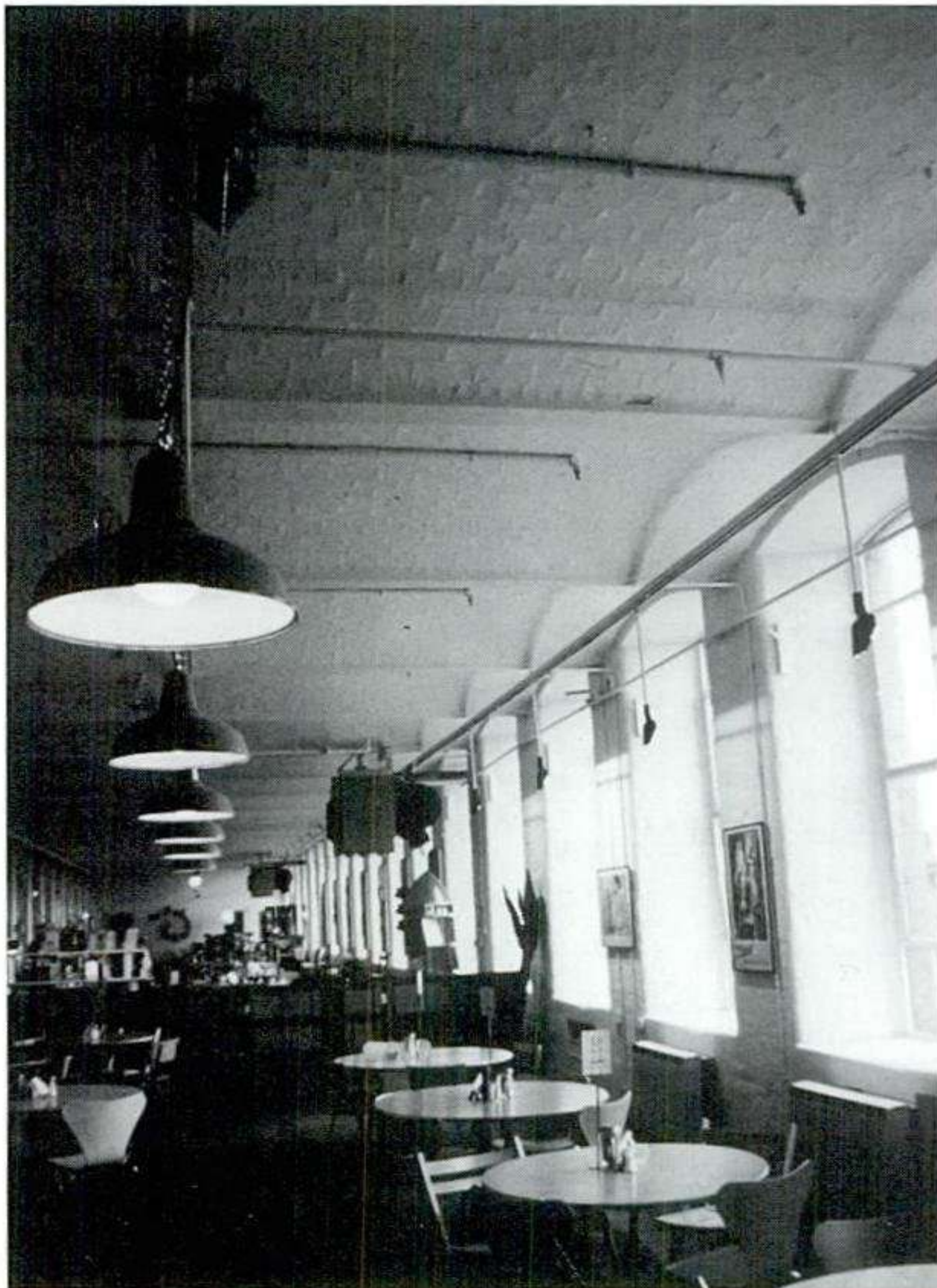
Fig. 16 Sprinkler installation. The historic uses of sprinkler systems in Britain tend to predominate in industrial and commercial buildings. This is, perhaps, not surprising. What is of interest in this case, where the original sprinkler installation was left in-situ following conversion of the industrial premises, it was not retained in an active mode!
