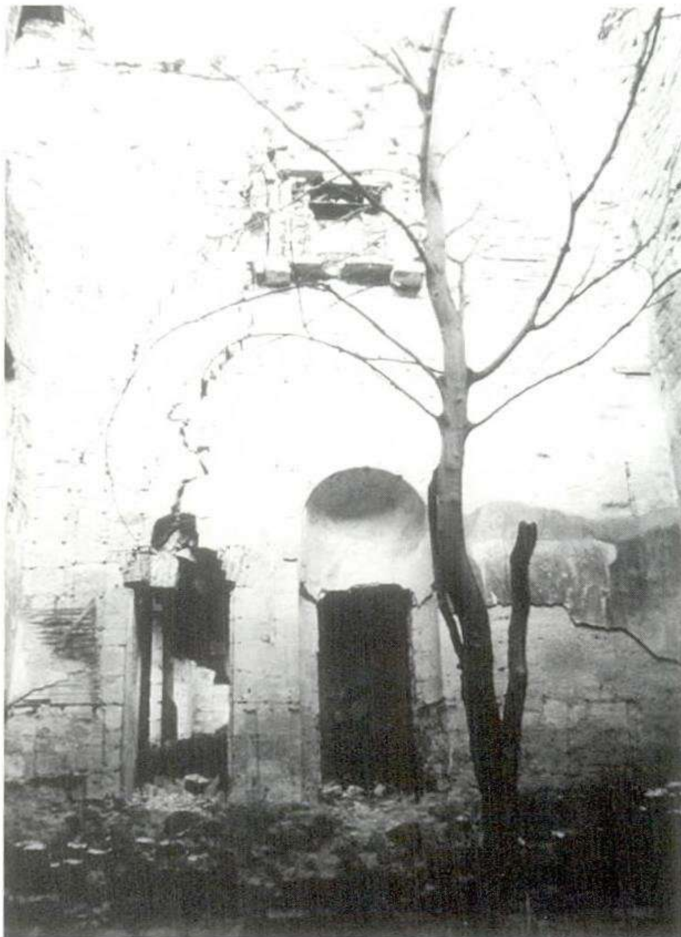
Fig. 2 Penicuick House. Although internal plasterwork fragments remain after 100 years of being roofless, nature has invaded the fire damaged interior. Structural disruption of the masonry has also occurred, with wallheads, chimneys, flues and openings being particularly vulnerable.
