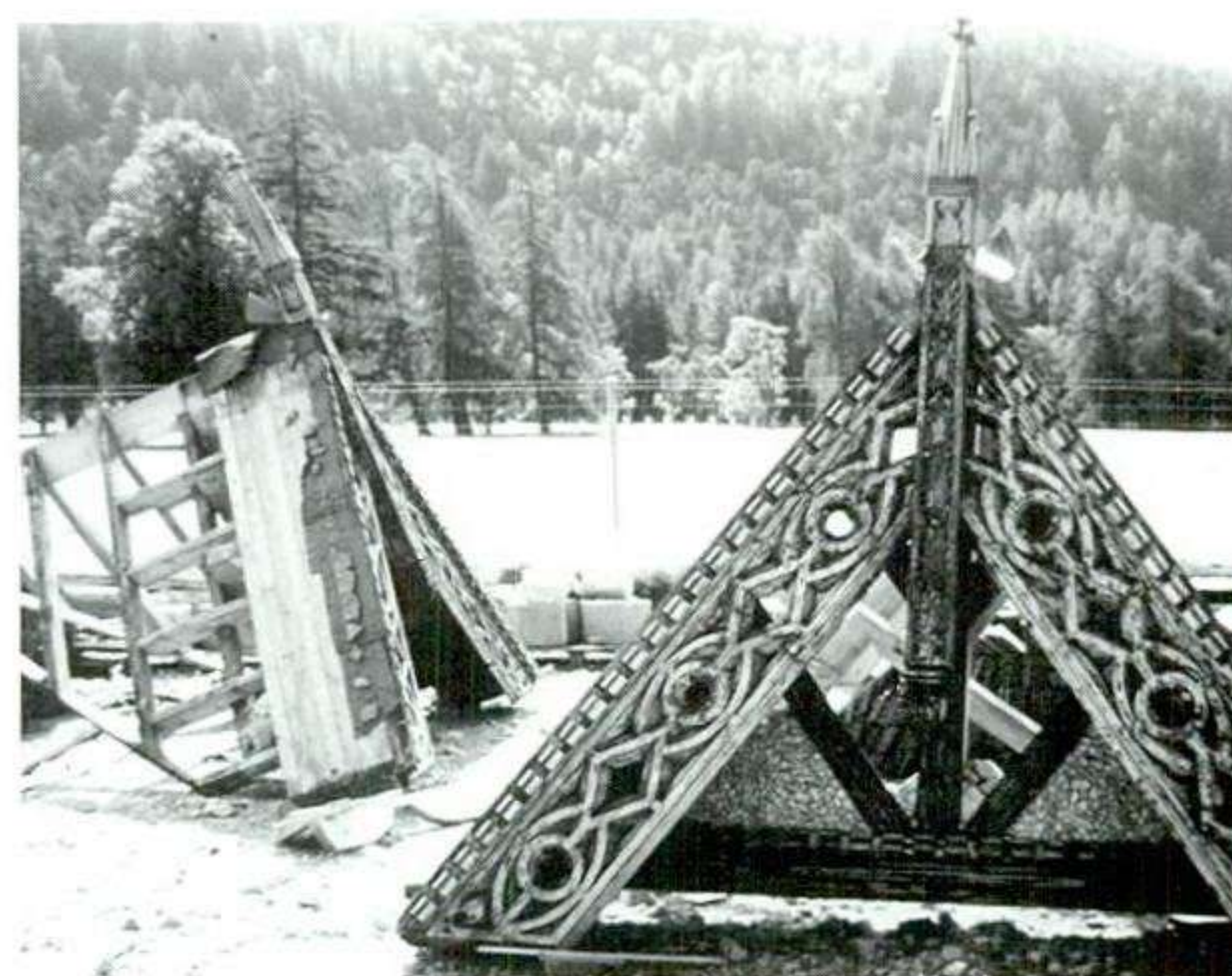
Fig. 15 Salvage. If no accurate records exist of a fire-damaged building, the period following a fire might be the only possible time to research the building's construction and finishes. Recording where burnt roof trusses and floor beams fell can assist in an accurate structural reconstruction of the premise, and the salvage of architectural features during an incident might allow their reuse.
