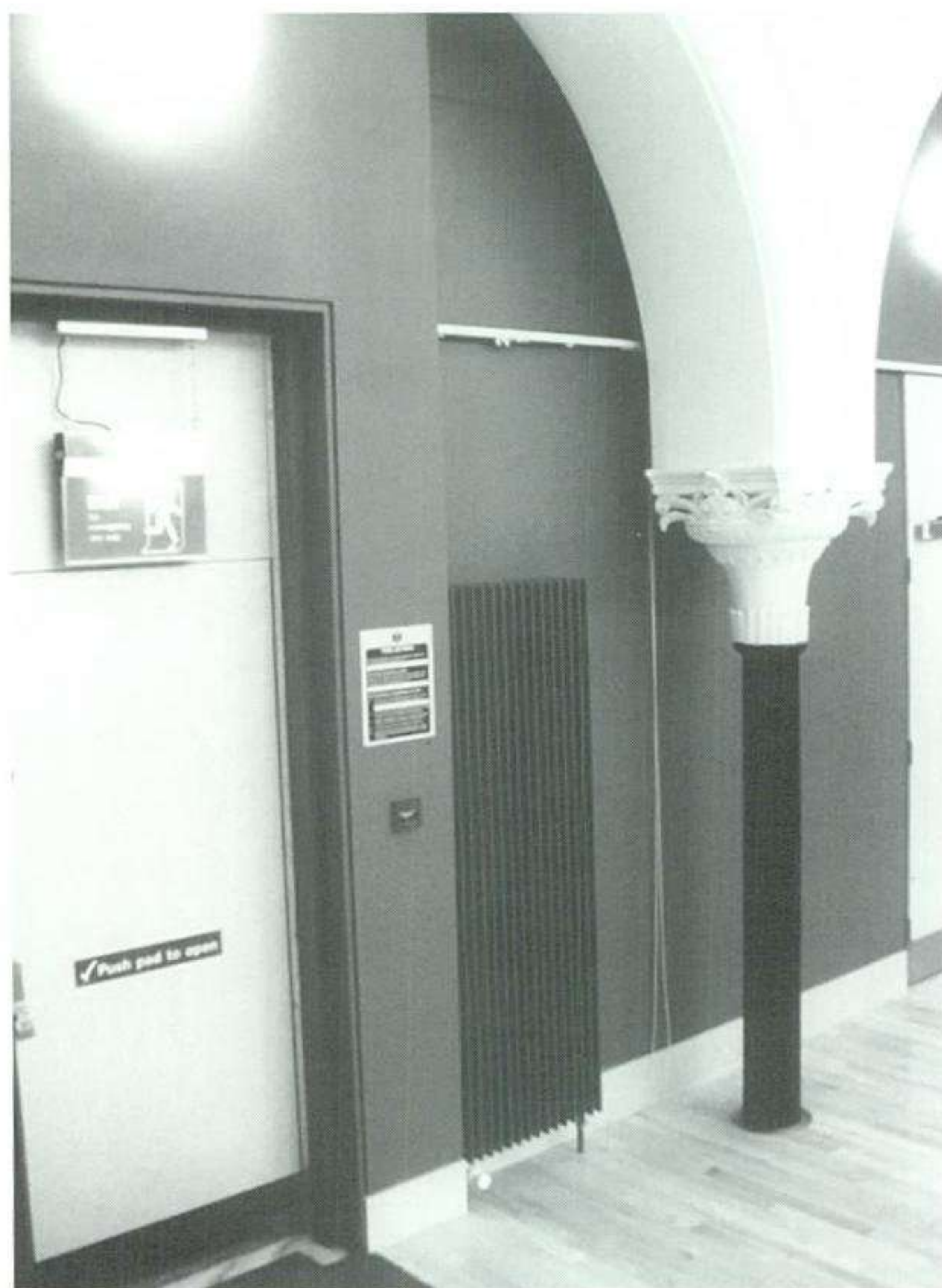
Fig. 14 Listed building adaptation. Through adopting an approach that separated the modern structure from the historic construction, a sympathetic conversion has taken place in this redundant church. However, the requirement to have a fire extinguisher, push-bar door-pad, pendent emergency lighting, fire alarm point and three stick-on instruction labels create a distracting, non-integrated appearance around the escape door.
