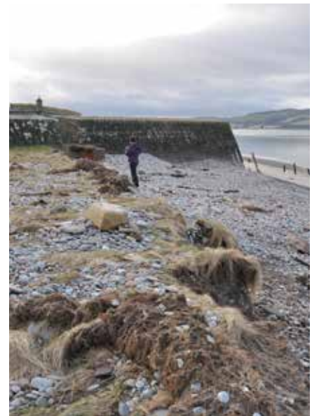
Figure 23: Damage to vegetation layer at Fort George as a result of winter storms (photo taken Feb 2013). In recent years it is not unusual for a metre of turf to be lost each year.
