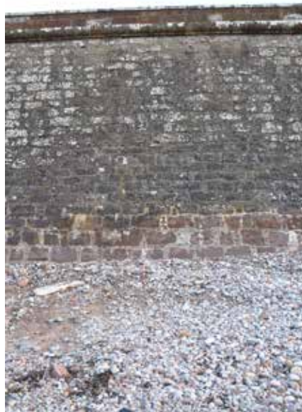
Figure 22: Part of Fort George sea wall showing 'clean' lower part where turf and soil layer has been completely eroded, leaving the masonry vulnerable to the sea.
