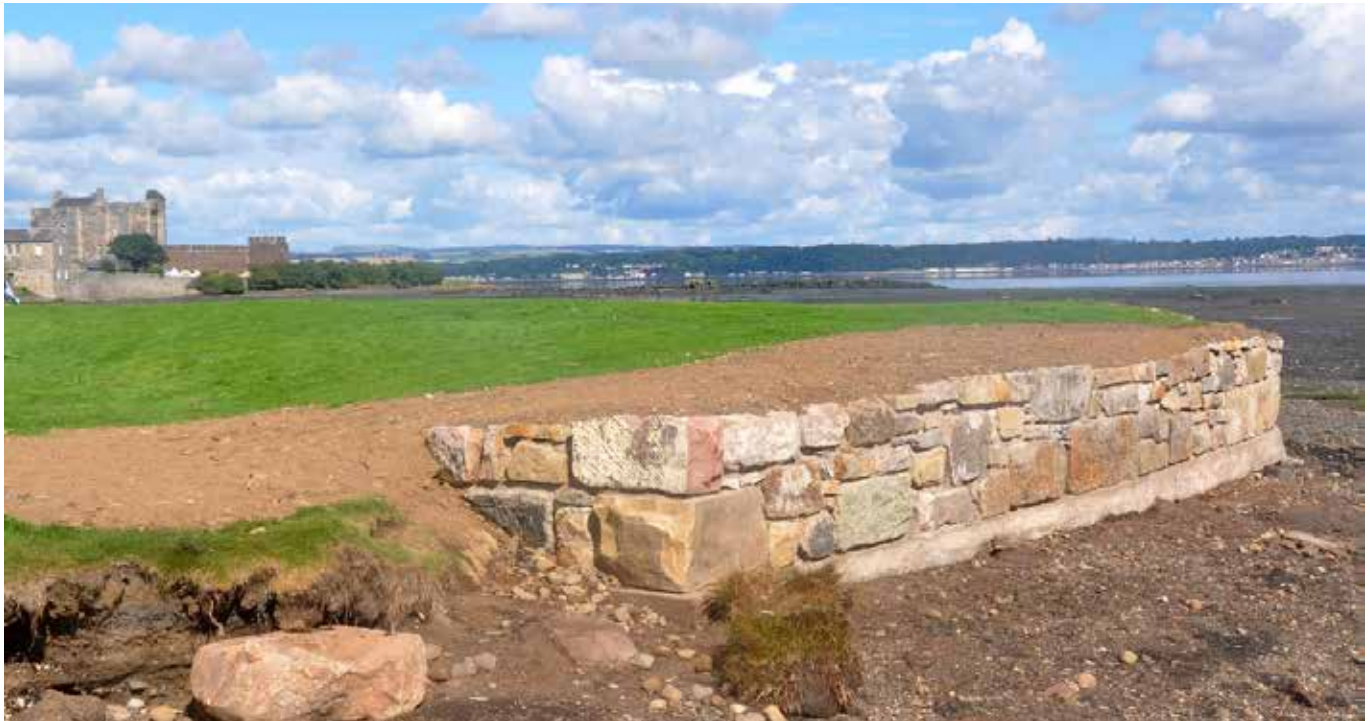
Figure 18: A newly constructed shore front wall at Blackness Castle. This helps protect the grounds behind from damaging wave action and coastal flooding.
