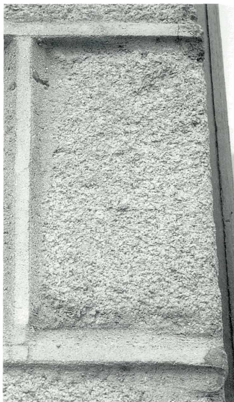
Plate 5 An example of re-pointing which has destroyed the visual impact of the granite. The granite is of the Loanhead type with a weathered and friable surface. The hard dense re-pointing will tend to increase the rate of decay of this granite.
