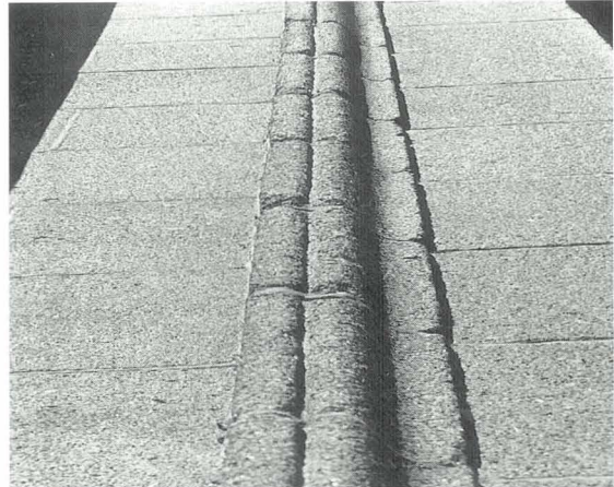
Plate 17 Part of arched opening John Smith Screen, Union Street, Aberdeen. The granite is Dancing Cairns and was cleaned by a chemical method 10 years previously. There is grain loss in association with the mortar joints. This elevation faces south to the street. The similar detail on the reverse of the arch (facing a church yard) remains intact.
