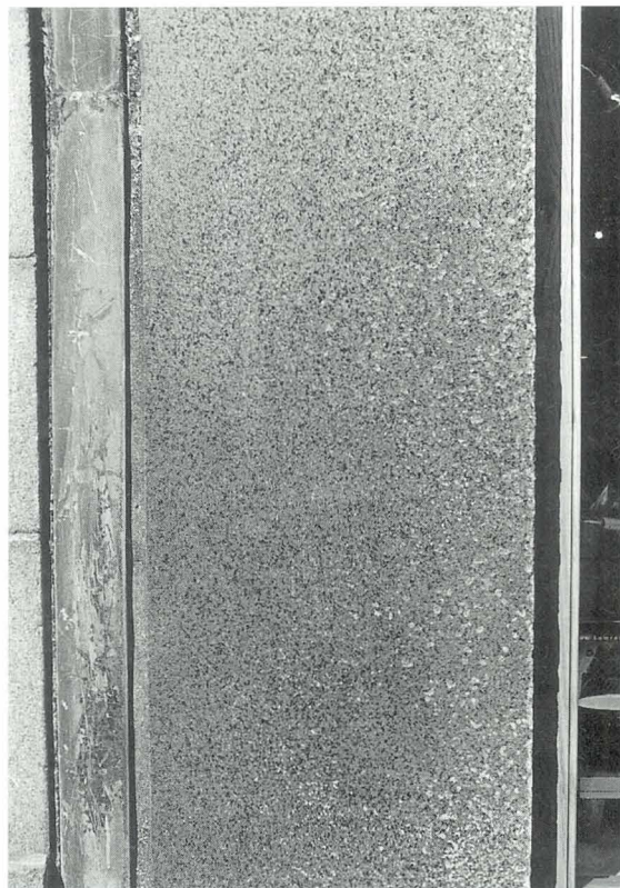
Plate 18 Granular disintegration on the surface of polished pink granite at city centre site. Cause unknown but may be associated with lack of proper protection during chemical cleaning of granite at a higher level on the facade.
