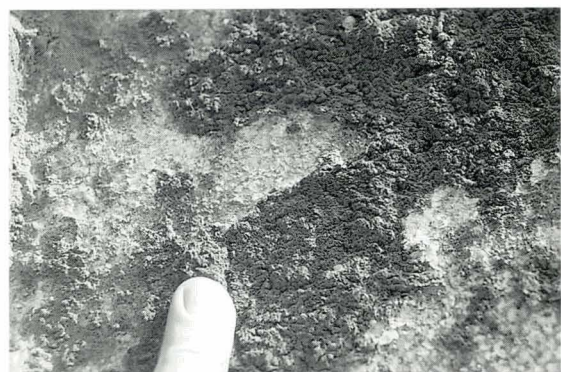
Plate 10 Close view of the soiling in Plate 9. The soiling is in a form of a hard gypsum crust, firmly bound to the granite. The crust is black due to the incorporation of hydrocarbons and other particulates into the gypsum.
