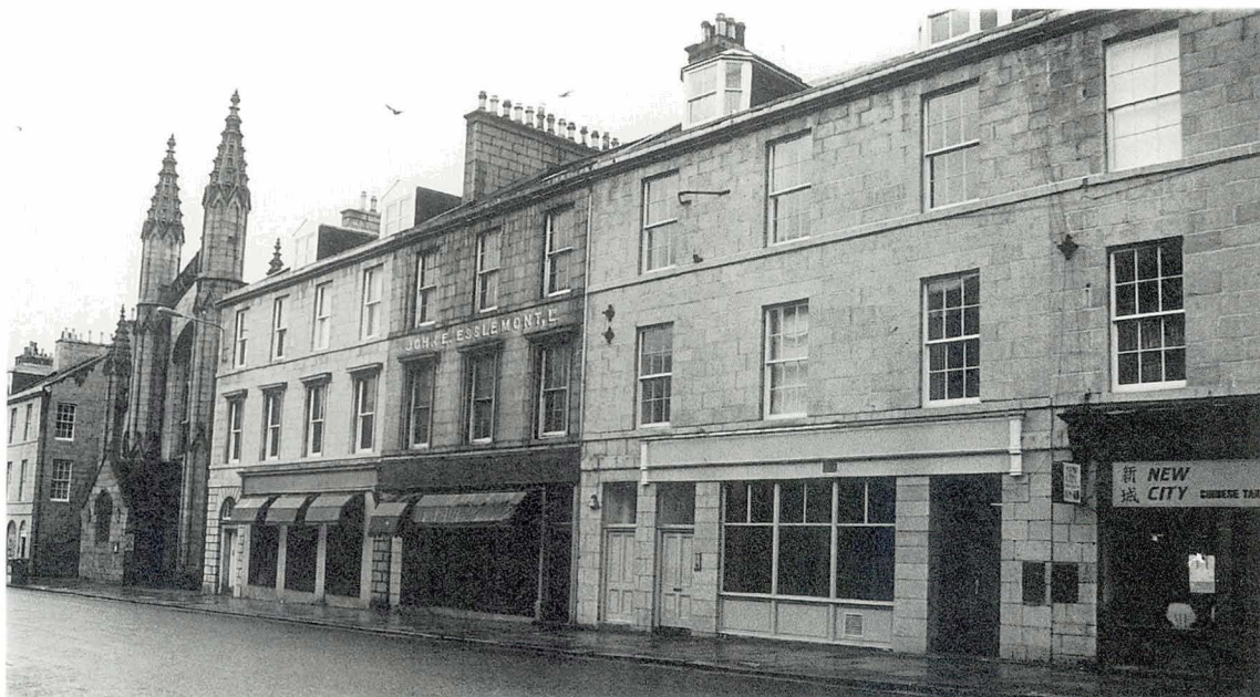
Plate 1 Patchwork effect of partial cleaning of a terrace (King Street, Aberdeen). Note the incomplete removal of soiling below the gutter. The dark patch to the right-hand side of the cleaned foreground building is a result of moisture being retained at decayed stone surfaces. The decay is not attributed to the wet abrasive (slurry) cleaning system which was used.
