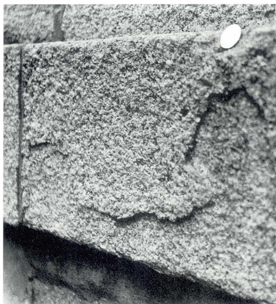
Plate 14 Contour scaling of projecting string course. Scales are several millimetres in thickness. Granite has been cleaned but method is not known.
