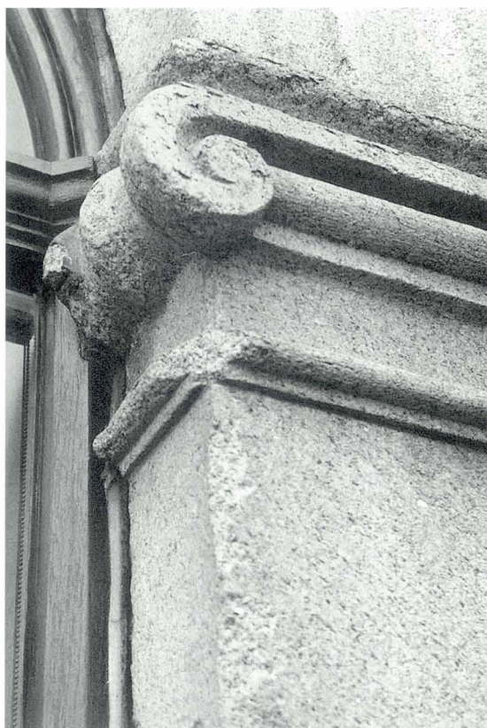
Plate 15 Scaling of cleaned Kemnay granite. Note the loss of detail on carved feature and at arrises.
