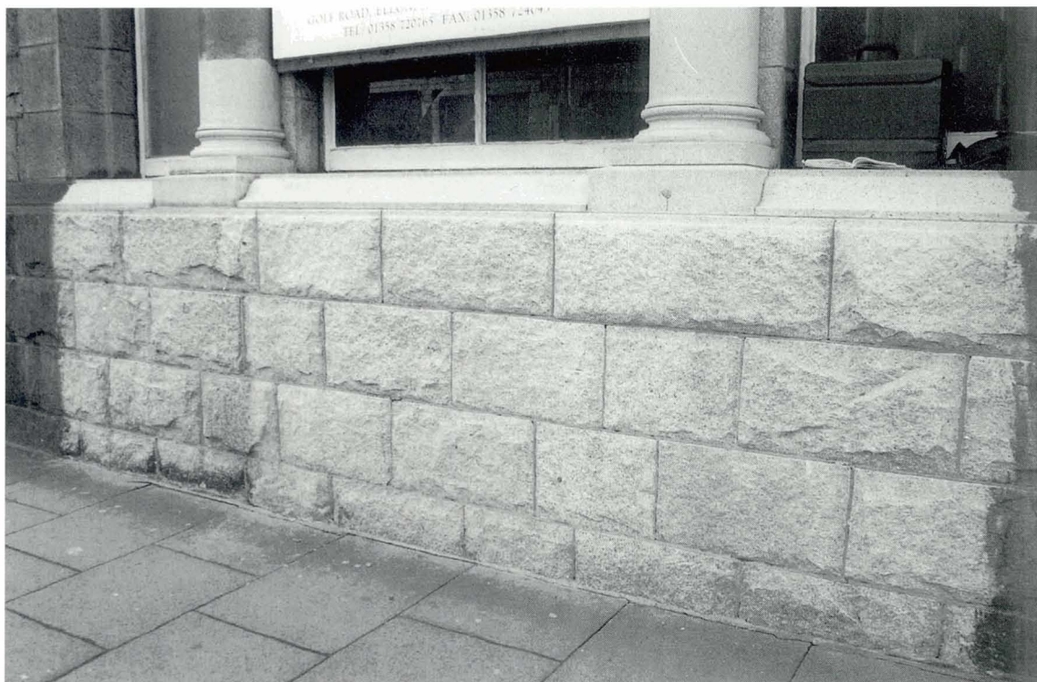
Plate 29 Test panels to assess three chemical cleaning systems for Listed Building Consent (Rubislaw type granite).
