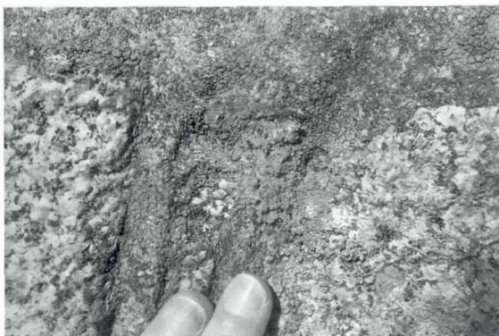
Plate 13 Lichen growths on Dalbeattie granite and on mortar joints. The presence of lichens is an indication of low levels of atmospheric pollution.
