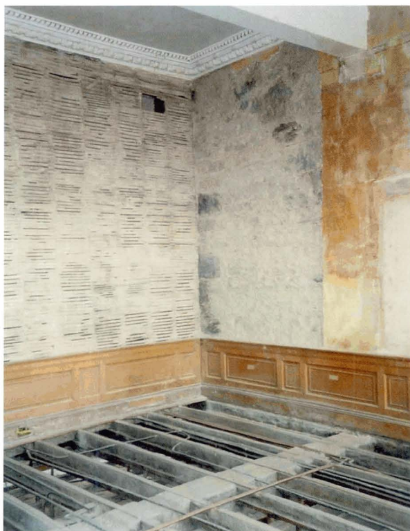
Illus 107 Stripping out of an interior during refurbishment work may provide a good opportunity to record wall and sub floor structures. This shows an interior in Charlotte Square, as it had been left prior to purchase by the NTS. (Photo: Ross Dallas)
