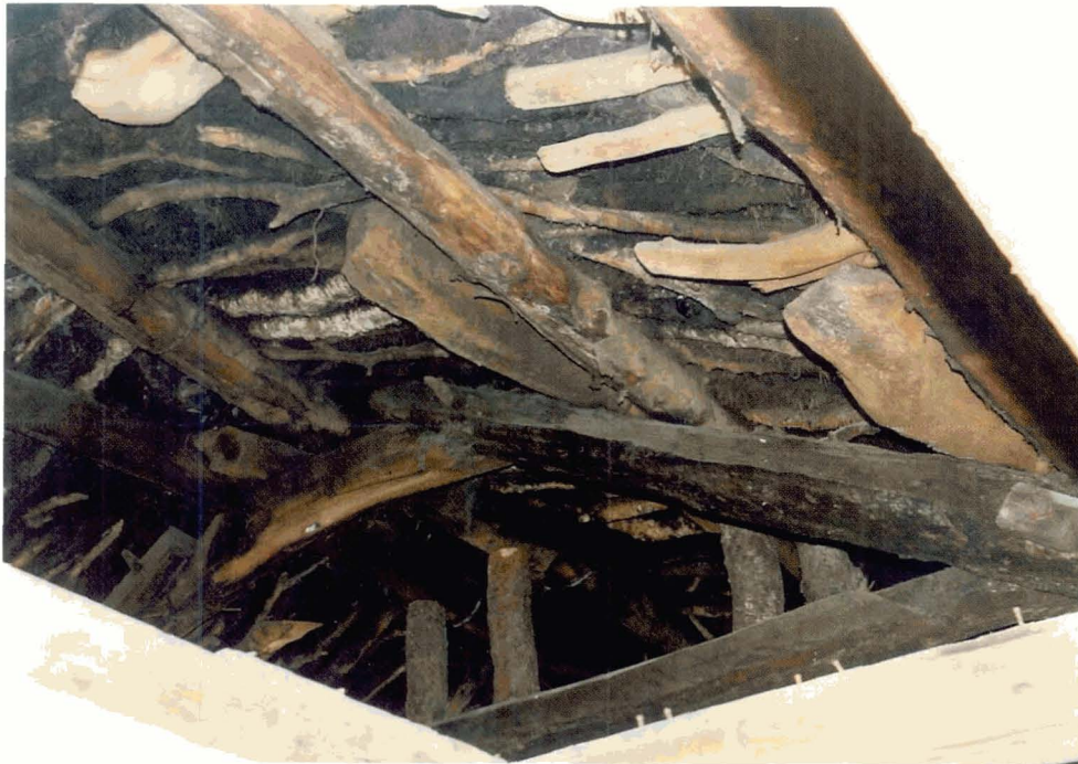
Illus 84 Timber roof construction in a dwelling, now covered in corrugated iron, at Auchindrain Township, Argyll. (Photo: Ross Dallas)
