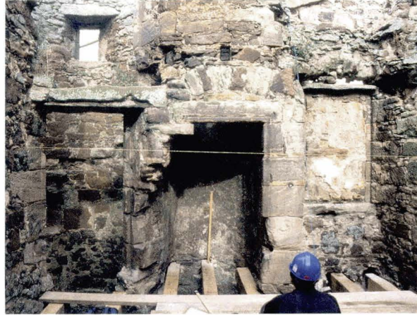
Illus 165 An internal elevation, with survey work in progress, east wing second floor. A horizontal datum line can be seen. Due to site conditions, much of the internal survey was carried out as the reconstruction work was in progress. New oak floor beams slotted into the original openings can be seen. (Photo: CFA Ltd)
