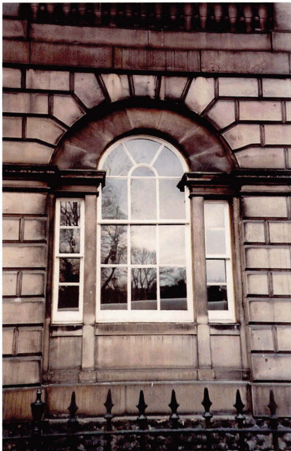
Illus 81 Ashlar stonework of the highest quality at Charlotte Square, Edinburgh (see Ch 1.8, for a drawing of this elevation). (Photo: Ross Dallas)
