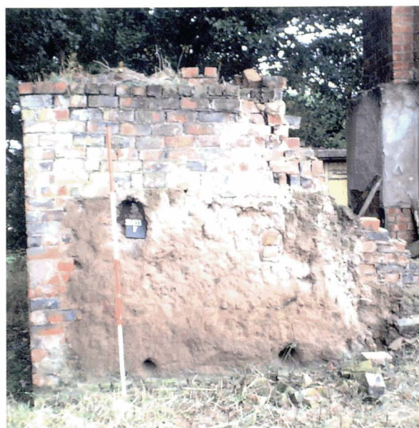
Illus 70 A typical view of an external wall, with the original clay construction built over with later materials. (Photo: SUAT)
