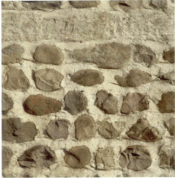
Illus 130 An area of well-preserved exterior rubblework pointing, where the craftsman's individual trowel marks are clearly apparent.
