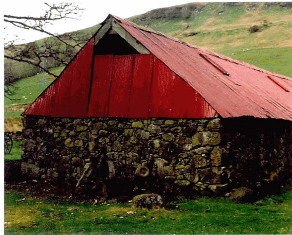
Illus 80 Random unmortared stone walling with corrugated iron above, used in the construction of a C19 barn at Auchindrain Township, Argyll. (Photo: Ross Dallas)
