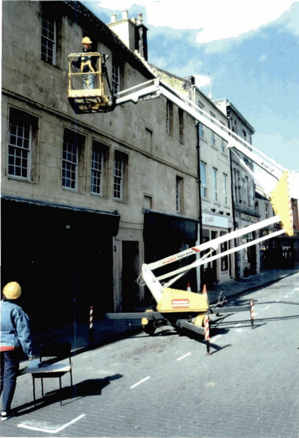
Illus 53 The front elevation of The Merchant's House, with survey in progress. An access platform or 'cherry picker' is in use. (Photo: Andrew Hollinrake/Kirkdale)
