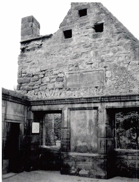
Illus 91 Panelling is most commonly found as a feature in woodwork, but here at the Dunfermline Aisle, Dalgety Bay, Fife, the detail is worked in stone. The former ceiling vault scar on the gable can also be seen on the right. (Photo: Historic Scotland)
