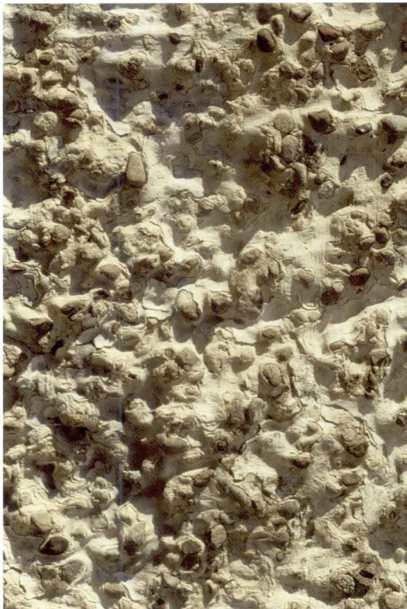
Illus 129 A detail of the same, illustrating the build-up of layers of limewash. Both illustrate the high aesthetic quality of the surface texture.
