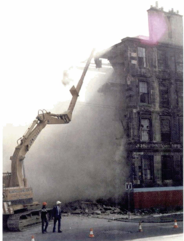
Illus 105 Demolition in progress!! This is emphatically what is not wanted – an uncontrolled demolition in this manner leads to the loss of a huge amount of invaluable historical evidence. (Photo: Ross Dallas)
