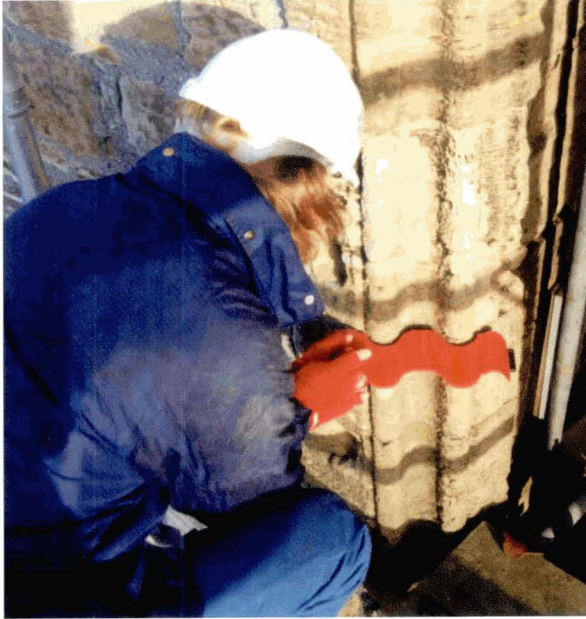
Illus 26 Utilising a profile gauge to record stonework detail. The gauge is gently pressed in against the stonework until it takes up the profile. (Photo: Historic Scotland)
