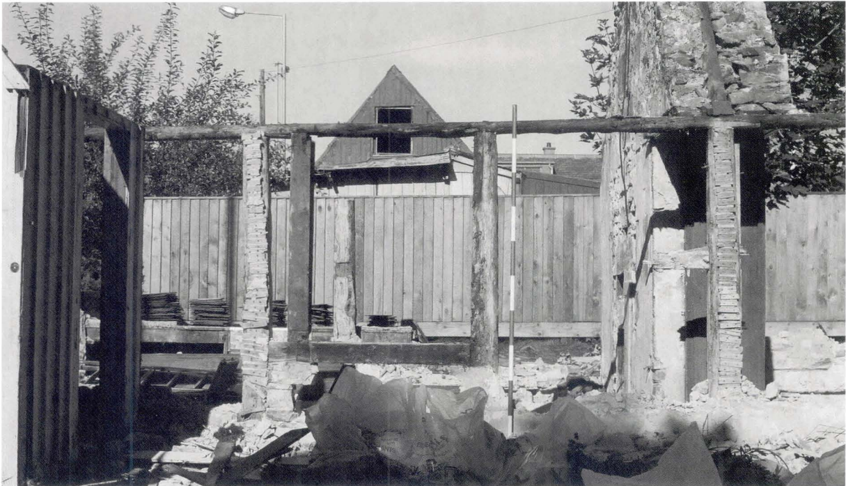
Illus 109 Dismantling of the cottage revealed that the construction was of far earlier date than apparent. (Photo: GUARD)
