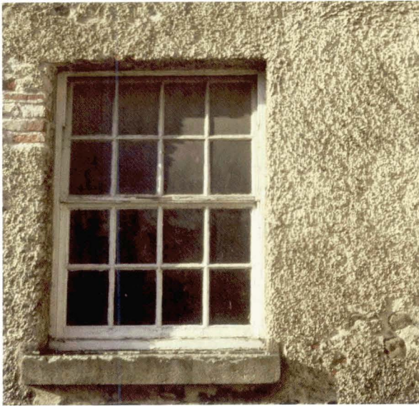
Illus 128 An area of historic harl of C18 date, where the individual casts from the harling trowel can be seen in the good cross-light.
