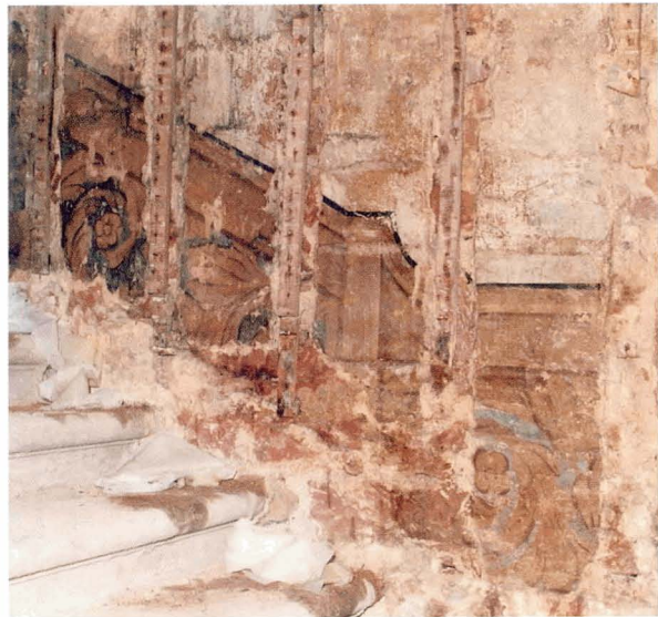
Illus 97 A survival of an earlier decorative scheme in Strathleven House. A later lath and plaster wall has protected an earlier painted trompe l'oeil dado. (Photo: Historic Scotland)
