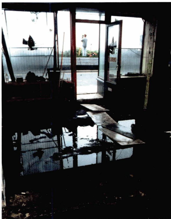
Illus 56 Ground floor interior of the former restaurant area, note flooding experienced after heavy rain. (Photo: Andrew Hollinrake/Kirkdale)
