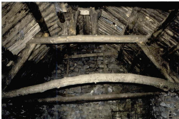
Illus 95 The roof of the long house at Moirlanich, Killin. The young, untrimmed timbers characteristic of vernacular buildings are visible. (Photo: AOC, courtesy NTS)
