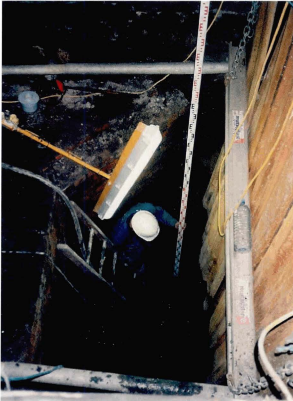
Illus 6 Excavation or 'dig' archaeology may often be essential. Here, archaeologists are excavating the area of a new lift shaft, Scotland Street School, Glasgow. (Photo and work: GUARD)
