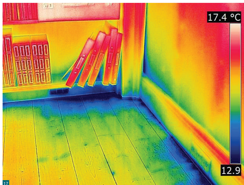
Fig. 17 The blue areas on the floor reveal a cold draught at the gap between skirting and floor. The wispy appearance of the chilled area is typical of the appearance of draughts on surfaces. The thermal camera cannot observe the cold draught itself, only its chilling effect on adjacent surfaces.
