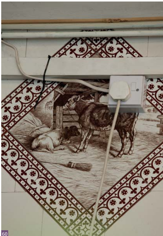
Fig. 60 Modern fittings such as electrics should not be installed where historic fabric can be damaged
