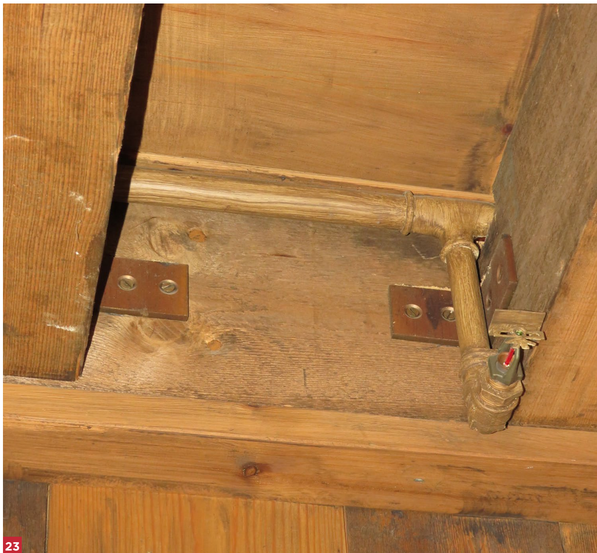
Figure 23. The sprinkler system at Corgarff Castle. The piping has been painted to match the colour of the surrounding timber.
