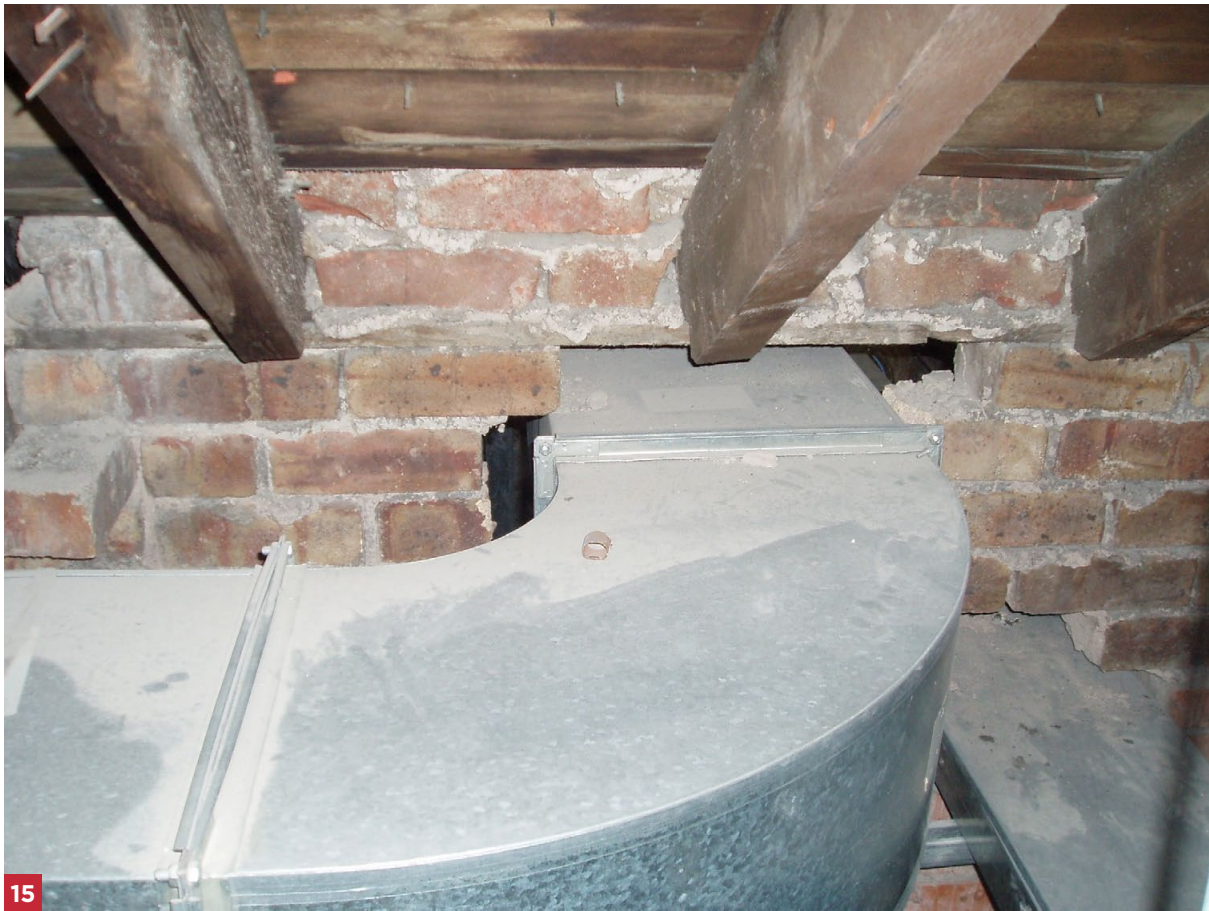
Figure 15. Poor fire compartmentation in a roof space.
