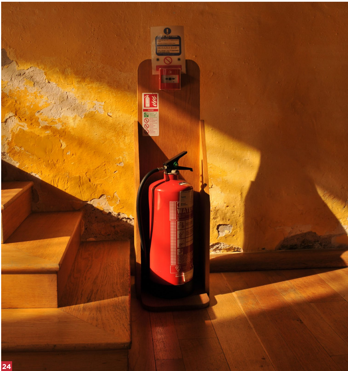
Figure 24. A fire extinguisher on a free-standing wooden base at Stirling Castle's Chapel Royal.
