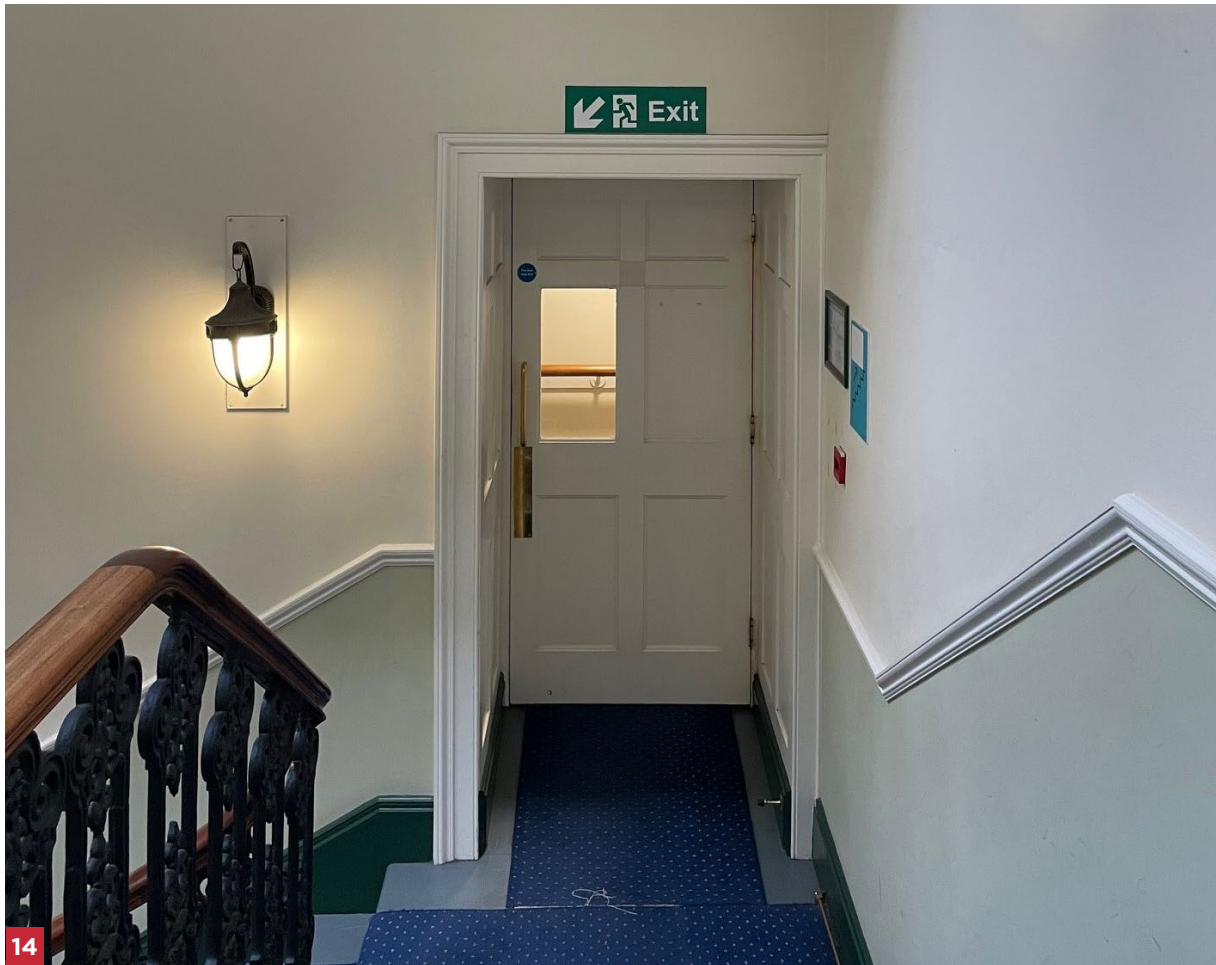
Figure 14. A new fire door onto an escape stair at a former hospital in Edinburgh that has been converted into offices.
