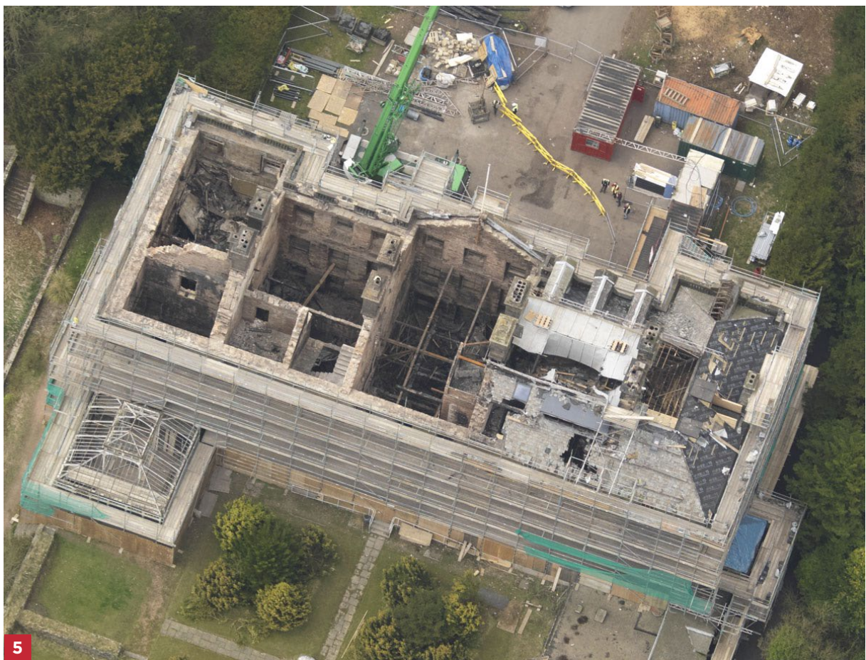
Figure 5. Leslie House in Fife suffered a serious fire towards the end of construction work in 2009.
