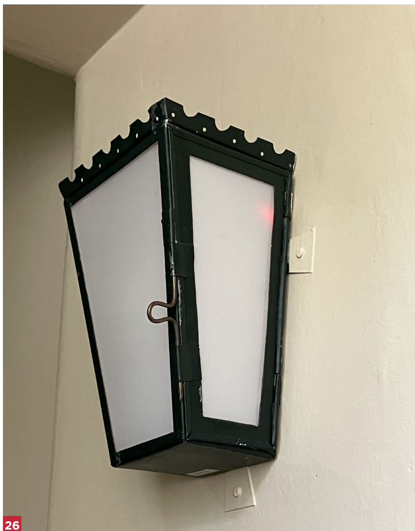
Figure 26. Discreet escape light fittings can be configured to suit a historic interior, as seen at Duff House.
