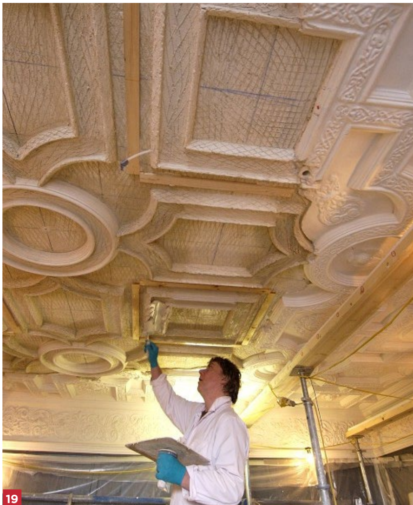
Figure 19. An aspirating smoke detection system was installed in the Laich Hall at Edinburgh Castle during restoration work. These systems draw air through small pipes to detect smoke. You can see the small white pipe here before it has been cut back to lie flush with the ceiling, forming a nearly invisible detection system.
