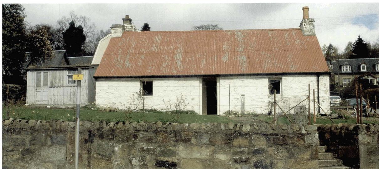
Illus 7 Sunnybrae Cottage, Pitlochry ©Bruce Walker. A corrugated iron roof was used to overlay and protect the underlying thatch
