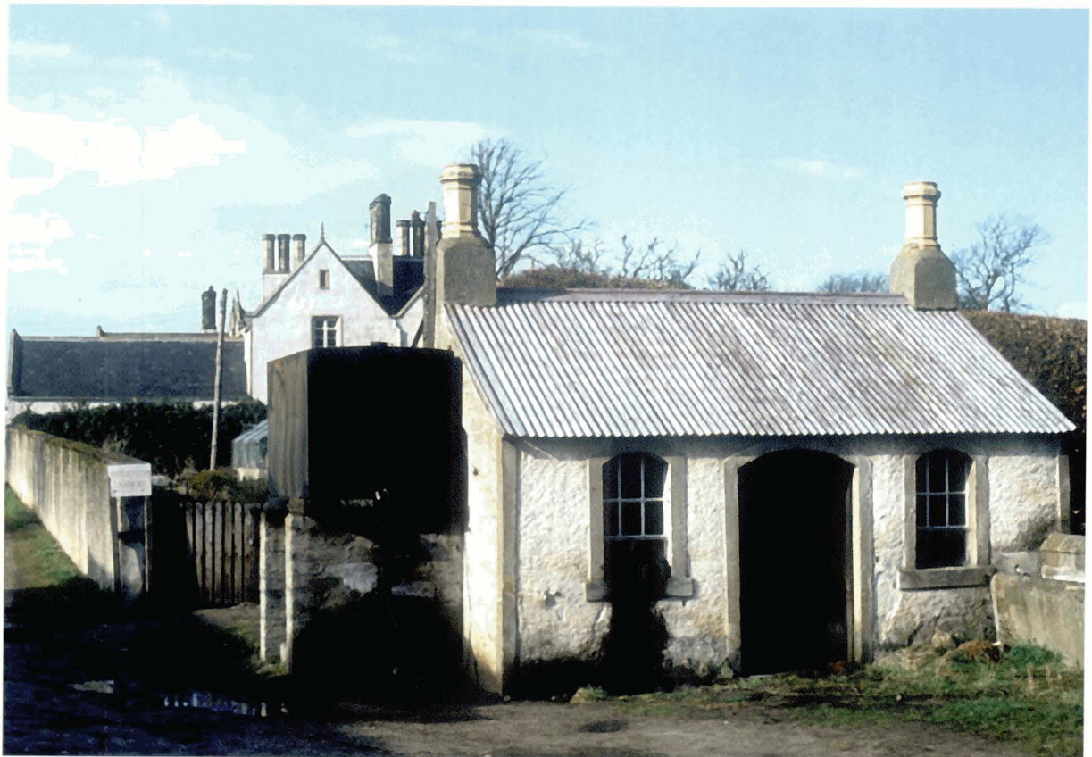
Illus 5 Sheriffston Farm Cottage, Elgin. Half roofed with single sheets of corrugated iron. © Ingval Maxwell
