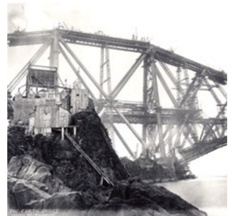
Inchgarvie north cantilever under construction in 1888. © Crown Copyright National Records of Scotland, BR/FOR/4/34/436.
