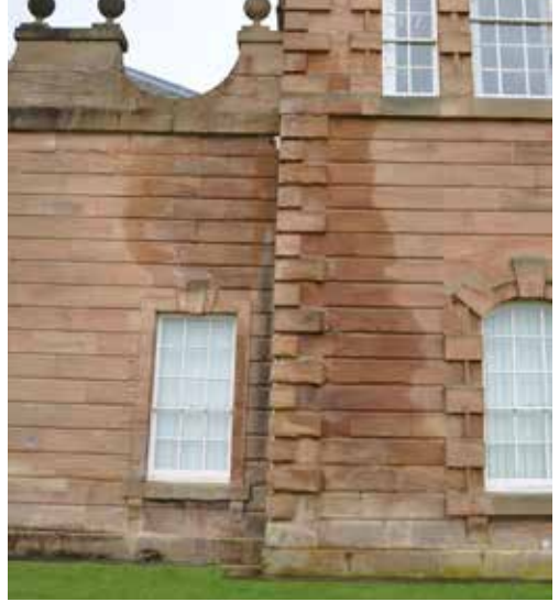
Fig. 3 Staining of masonry showing a blockage in the gutter behind this parapet.
