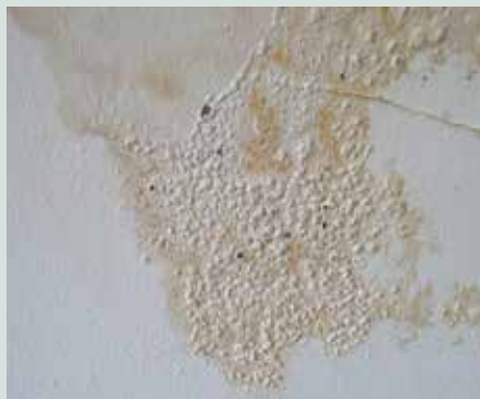
Fig. 1 Damp in a wall showing as blistering of this painted surface.
