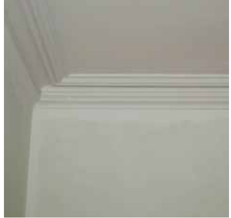
Fig. 9 The use of breathable materials will help ensure defects do not remain hidden; this ceiling has been painted with a modern clay-based paint.
