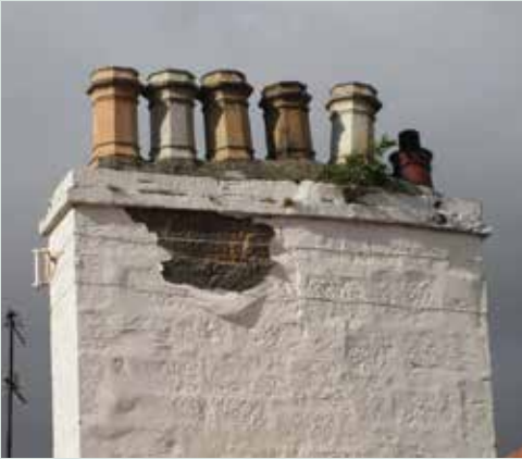
Fig. 4 The poor condition of this chimney has resulted in dampness internally.
