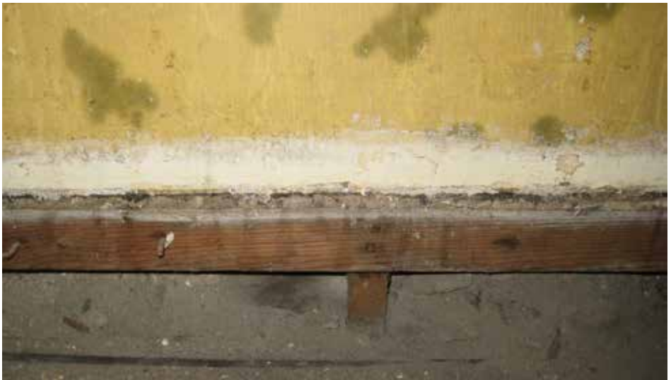
Fig. 8 The removal of a vinyl wallpaper and skirting board allows the wall to dry out and debris to be cleared.
