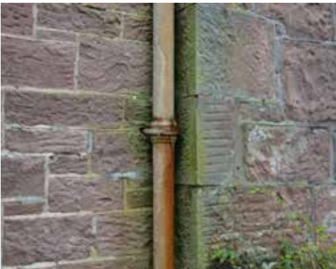
Fig. 2 A blocked downpipe causing saturation of the adjacent masonry. Plant growth is indicative of a saturated wall.
