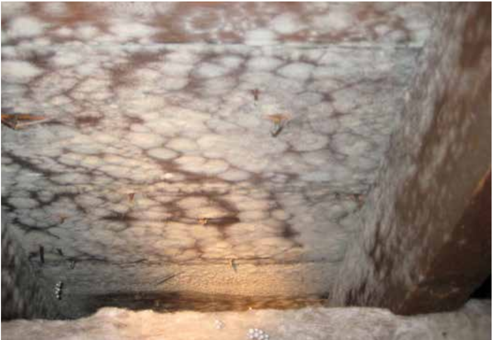
Fig. 10 Mould growth in an attic following insulation works; proper ventilation will prevent this.
