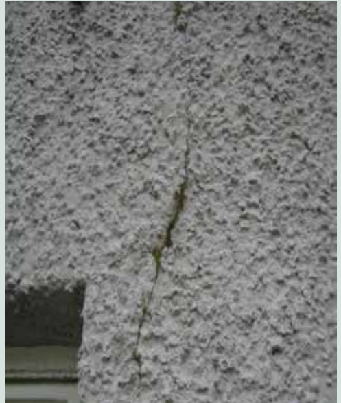
Fig. 5 Moss growth in cracks in this cement render indicate saturated masonry behind.
