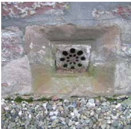
Fig. 6 A sub-floor vent; note the appropriate height and finish of the ground level.
