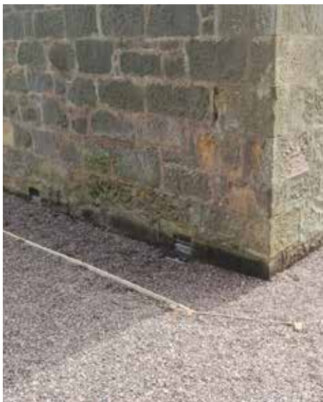
Fig. 7 Lowered ground levels and the clearing of the sub-floor vents during the refurbishment of this 19th-century cottage has resolved the damp problems in the walls.
