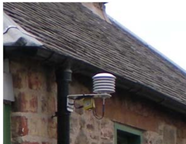
Figure A6. Tinytag Standard Thermistor Probe in a radiation shield tied to a rainwater downpipe. The probe is connected to a Tinytag Plus 2 data logger hanging from the shield bracket.
