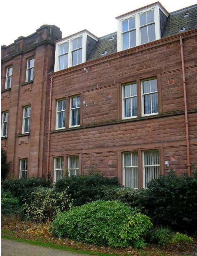
Figure 7. McCowan House (ID13) with several external ventilation grilles visible at high level either side of the windows.
