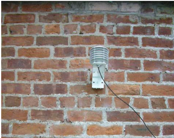
Figure A5. Campbell Scientific 107 Temperature Probe in a radiation shield screw-fixed into a mortar joint of the external wall face. The probe is connected to a data logger inside the building.
