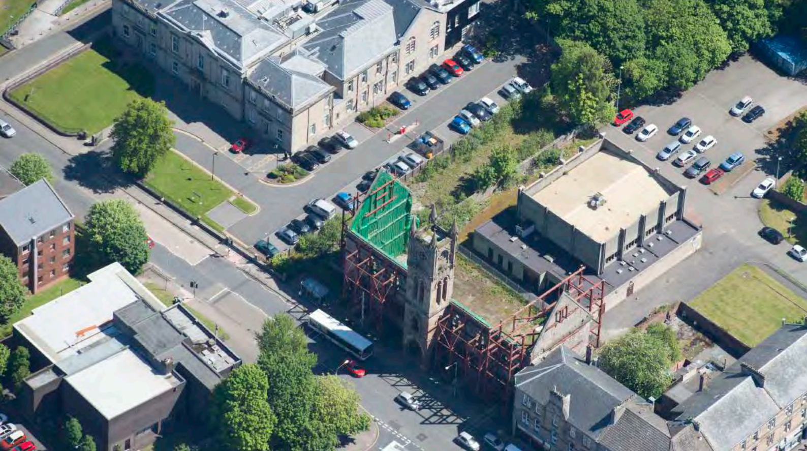
Above: Aerial view of Dumbarton Academy and Burgh Halls held up by a steel frame prior to the refurbishment project in 2015
