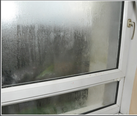
Fig. 1: Surface condensation is most often seen on windows; this can be a problem on both double and single glazed windows (Copyright MERU).
