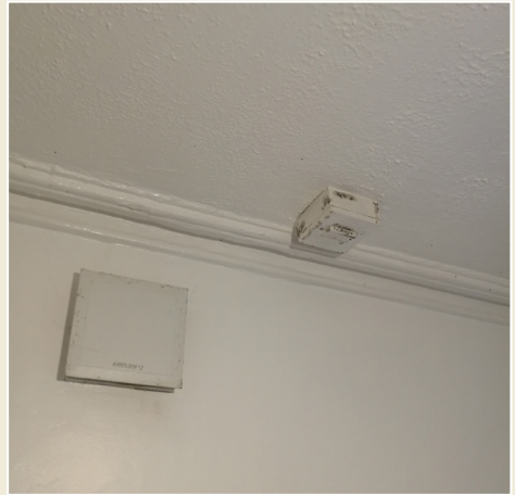
Fig. 4: Inadequate extract ventilation can be ineffective at removing condensation from buildings.
