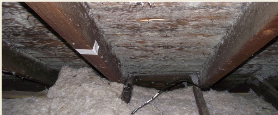
Fig. 5: Where lofts are insulated this reduces the temperature of sarking boards therefore raising the risk of condensation forming on the colder surface. This can lead to mould growth as seen in this image.
