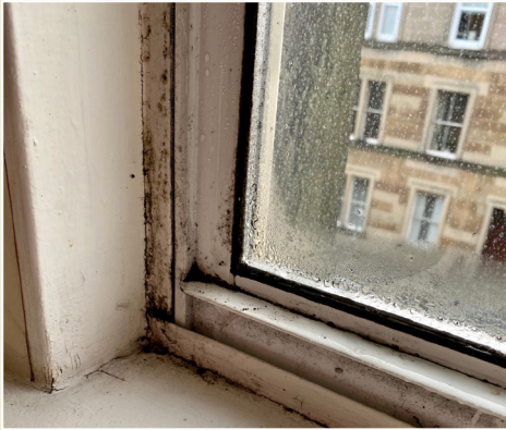
Fig. 2: Surface condensation can lead to decay of adjacent building elements; here, the condensation on the window is causing mould and decay to its timber surround (Copyright Glaze and Save).
