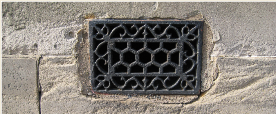
Fig. 6: External ground level vent: maintaining ventilation is one of the most effective means of reducing condensation risks in traditional buildings.
