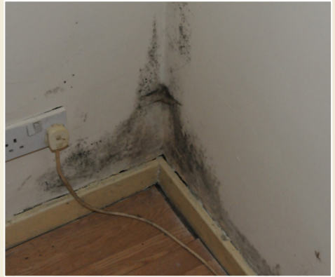
Fig. 3: The moisture created by condensation can lead to mould growth on building fabric (Copyright MERU).
