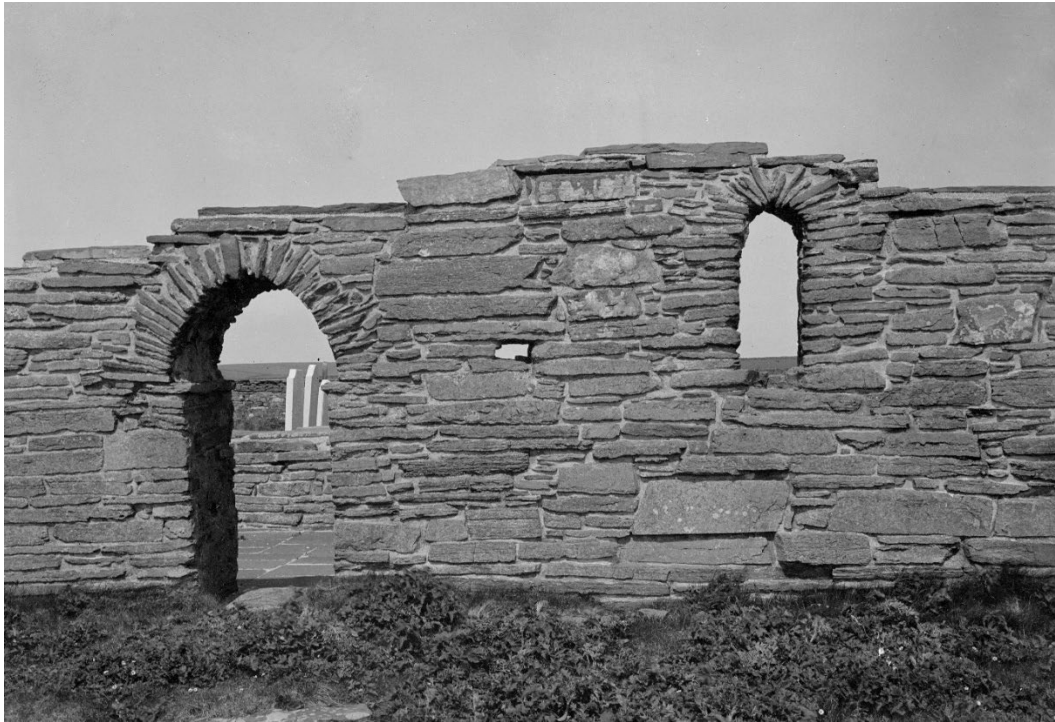
Figure 3: Entrance and round-arched window, with possible put-log socket in centre of image. Image c.1930, looking north. © Crown Copyright: HES.
