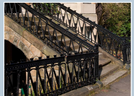
Circa 1865 cast-iron railings at a tenement in Sanda Street, Glasgow. © N. Haynes.
