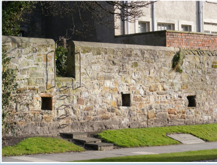
Three early 17th-century charter boles (used for defining boundaries and keeping property charters) set in the high wall of one of the long rig plots in South Street, St Andrews.
