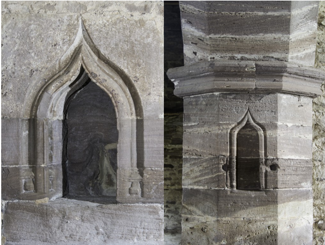
Figures 4a and 4b: Ogee-arched recesses in a) east end of south wall of chancel and b) east respond of south transeptal arch.
