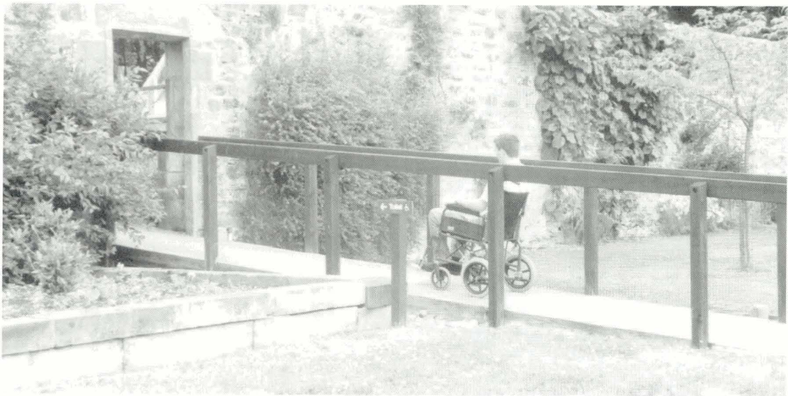
Plate 3. Fyvie Castle - Permanent ramp installation Note: Handrail is mounted too high and there are no guard or tapping rails.
