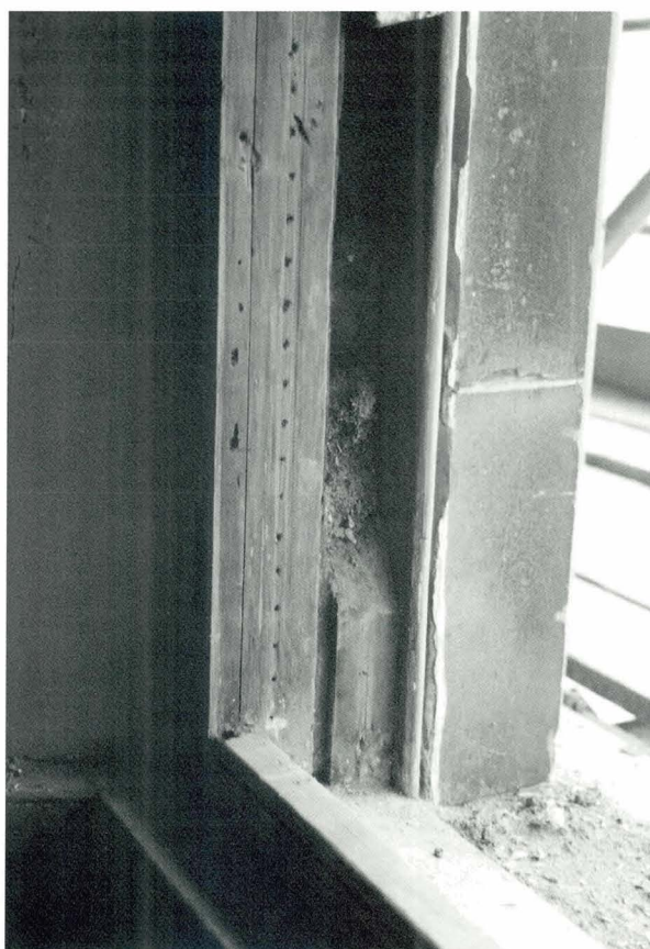
72 Weight pocket before repair.
