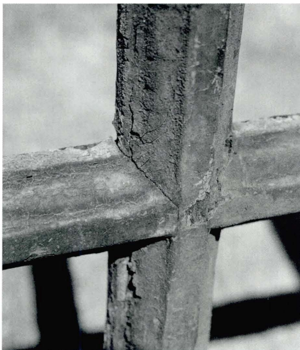
79 Layers of paint on an old window.
