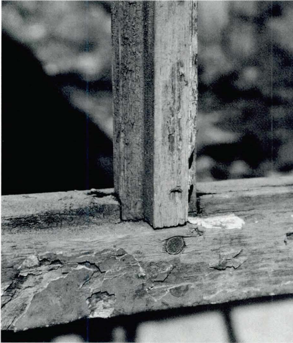
68 A loose sash joint.
