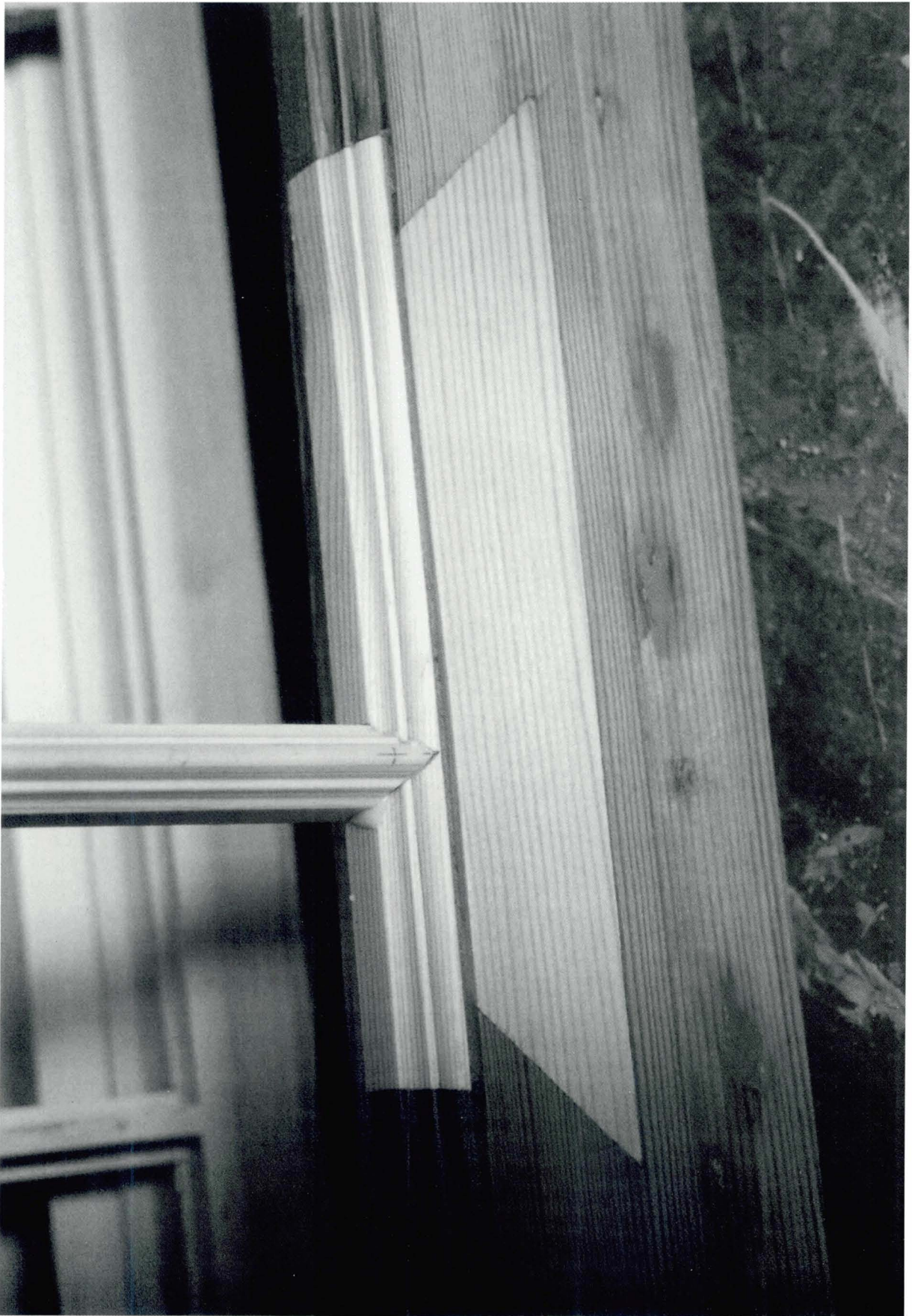
66 Replacement timbers to match those being replaced. Note the grain density and direction.
