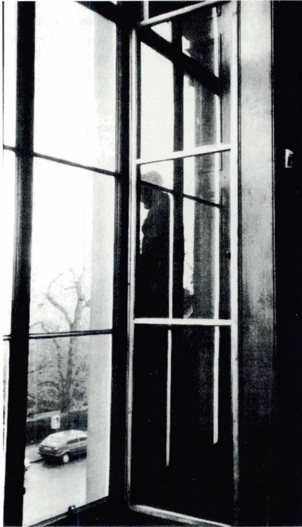
61 Original nineteenth century casement secondary glazing to sash and case window. Library, Royal College of Physicians, Edinburgh.
