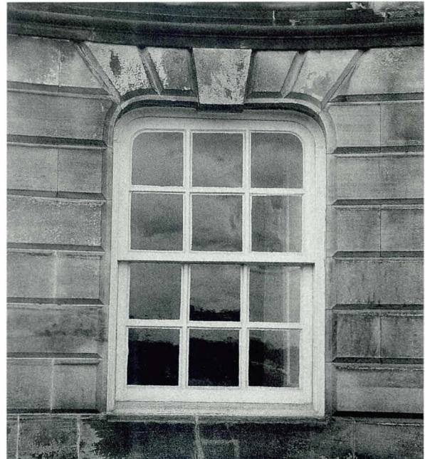
19 Basket arched window in the ground storey at Hopetoun, West Lothian. (Remodelled William Adam, 1721-48)
