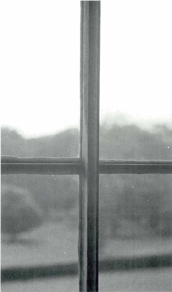
41 Very slender segmental metal glazing bar, tongued into vertical oak bar of normal early C19 proportions, at Abbotsford, Borders.
