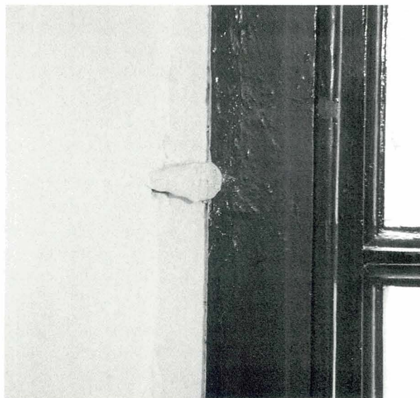
11 Wrought iron holdfast visible in a late C17 window without any internal covering joinery.
