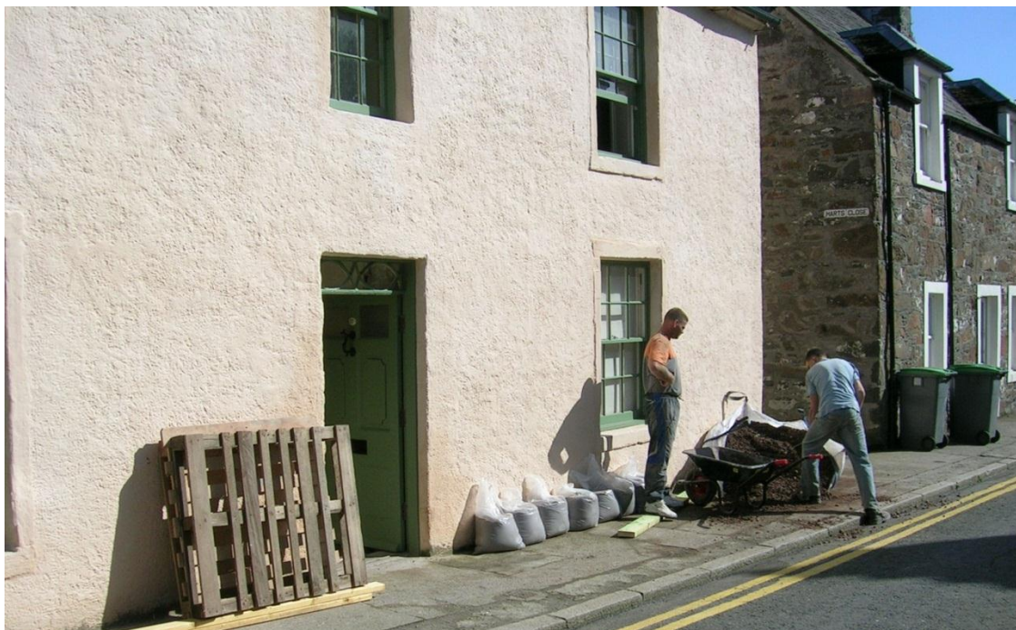
Fig. 11: A portion of the front facade after application of the lime harl.
