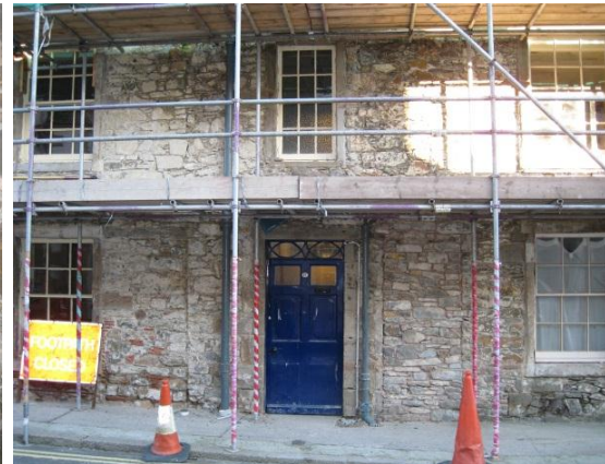
Fig. 10: Entry door to no. 29 is in-filled with stone, to the right of the existing entry door
