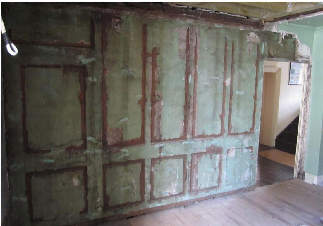
Fig. 25: Staircase removal from the first floor revealed a wood panelled wall behind
