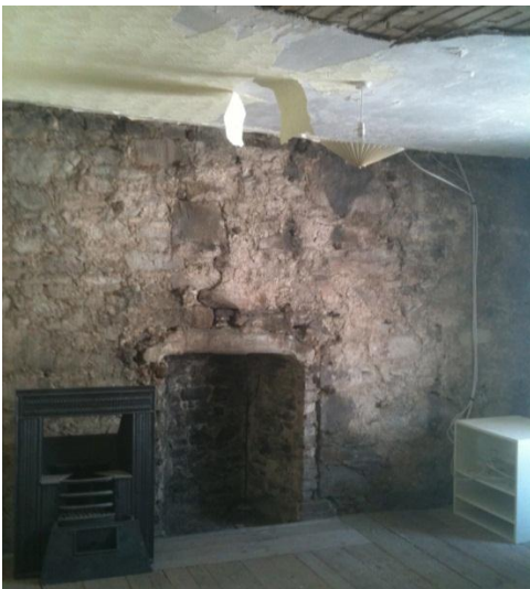
Fig. 28: Existing hearths were retained in all rooms, but were either plastered over or a fireplace was reinstated.
