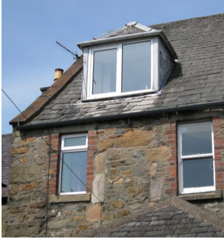
Fig. 38: The original opening for the bathroom can be seen between the two windows. These two later windows were removed and in-filled, and the original window reinstated.
