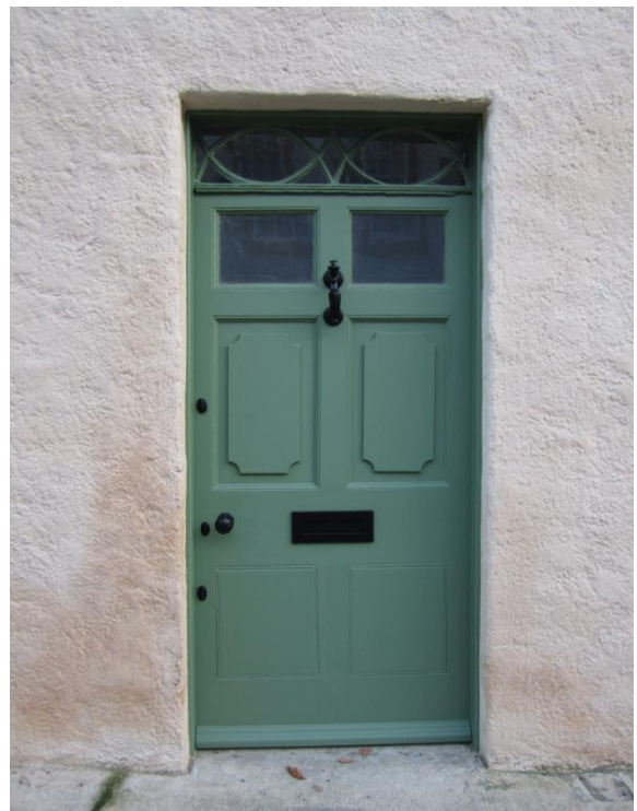
Fig. 22: The front door after refurbishment, with an improved drip rail across the bottom
