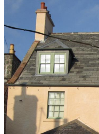
Fig. 40: Window reinstated at a higher position than the original window in this location
