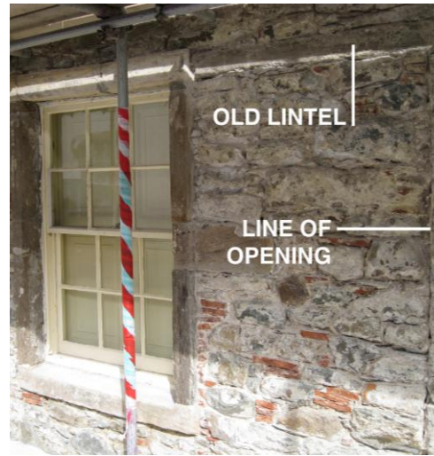
Fig. 4: Remnants of old shop door on front elevation
