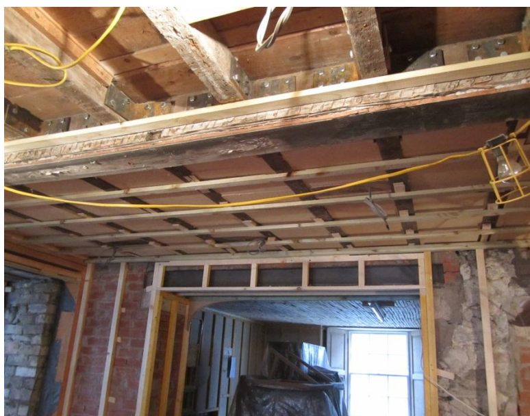
Fig. 37: Wood fibre insulation board installed in ceiling space above the dining room serves as acoustic and thermal insulation.
