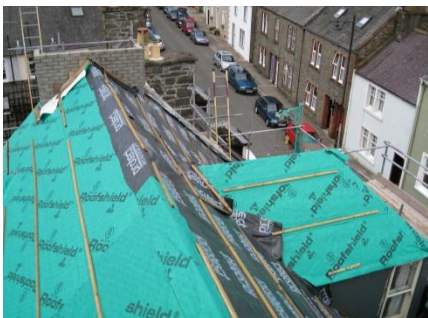
Fig. 6: Roofing membrane installed on roof after it was stripped of its slate.
