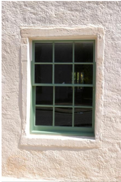
Fig. 19: New Georgian style window on front elevation, constructed from a template based on existing windows. Note the aged appearance of the stone surround is maintained.
