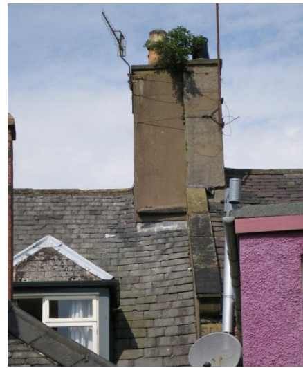
Fig. 14: North chimney, in line with chimney of adjoining property, prior to repair.
