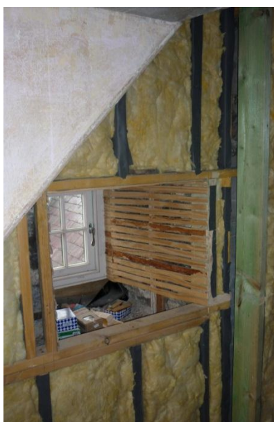
Fig. 36: Mineral wool insulation installed between studwork prior to application of lath and plaster
