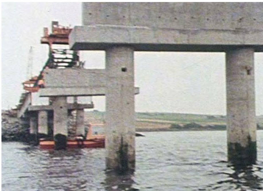
6 Still from the 35mm, colour film Cromarty Bridge , 1979, made for Films of Scotland and Fairclough Construction . Courtesy of Scottish Screen Archive at National Library of Scotland, ref 3054.
