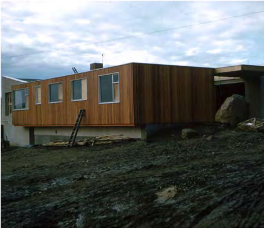
5 Robert Matthew's Gogarbank House (now Suntrap Centre) seen under construction in 1956. © RMJM
