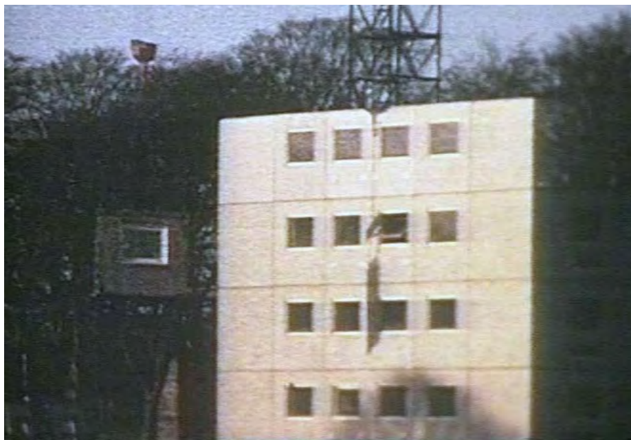
5 Tenement under construction at Trottick, Dundee, frame enlargement from the silent, 8mm, colour film Bett Homes. Courtesy of Scottish Screen Archive at National Library of Scotland, ref 5761
