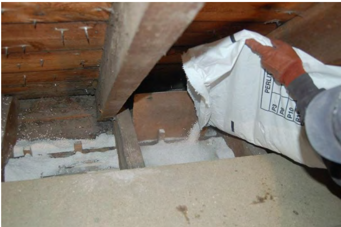
Figure 4: Pouring perlite insulation into wall void from the attic space at Scotstarvit Cottage (photo courtesy of Historic Environment Scotland).
