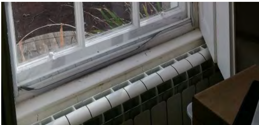
Figure 23: Failing magnetic strips on bottom sash rail around the secondary glazing at Wells o' Wearie.
