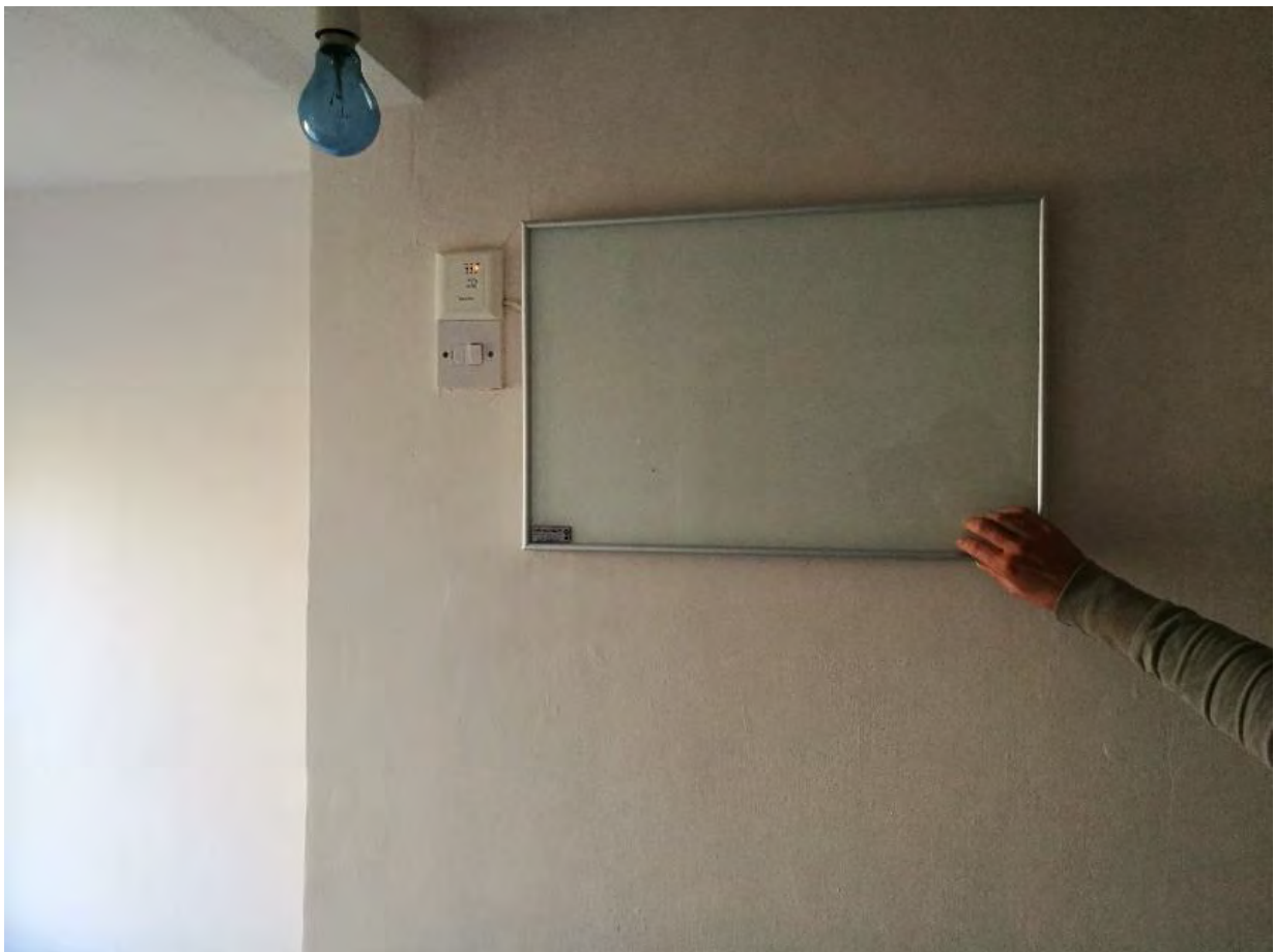
Figure 27: One of the heating panels used at Scotstarvit Cottage.
