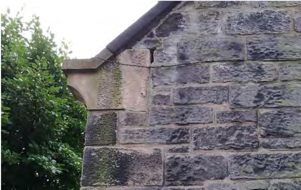
Figure 33: External masonry at Wells o' Wearie. The performance of the new wall insulation is being compromised by poor maintenance and inappropriate repairs resulting in damp walls which are less thermally efficient.
