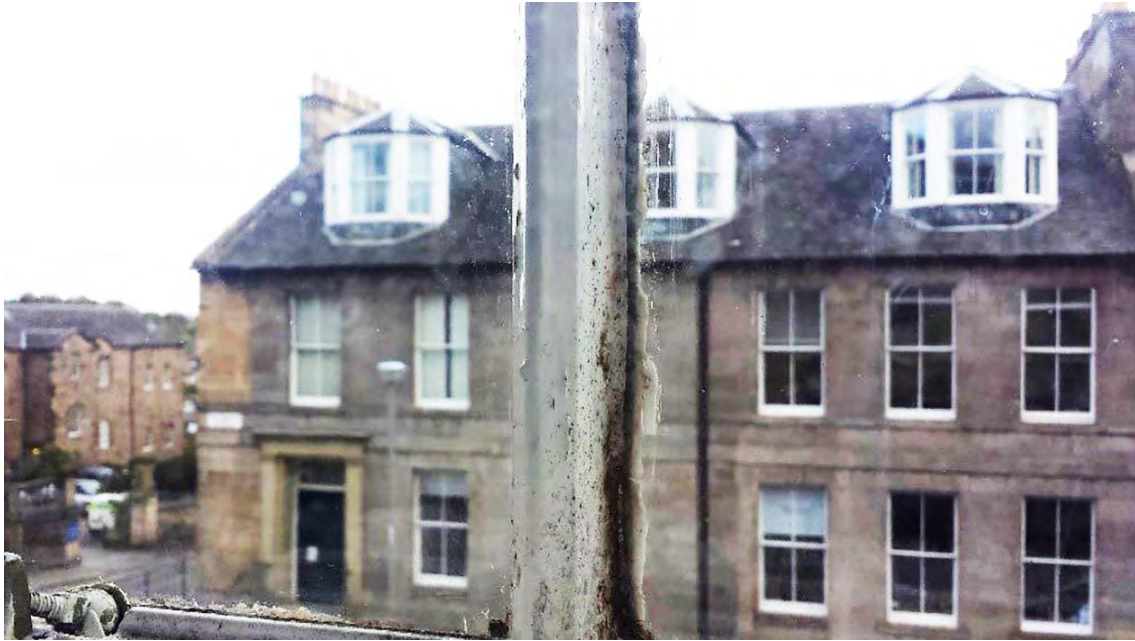
Figure 22: Mould growth on the windows of one of the tenement flats upgraded in Edinburgh, likely due to a lack of ventilation.
