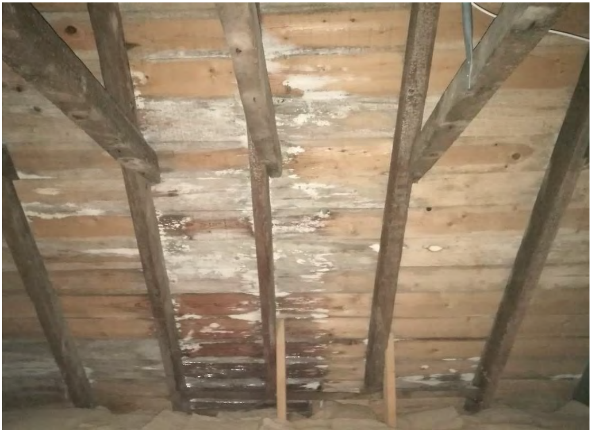
Figure 12: Mould visible on underside of sarking boards in an unventilated roof space following installation of insulation at Wee Causeway.
