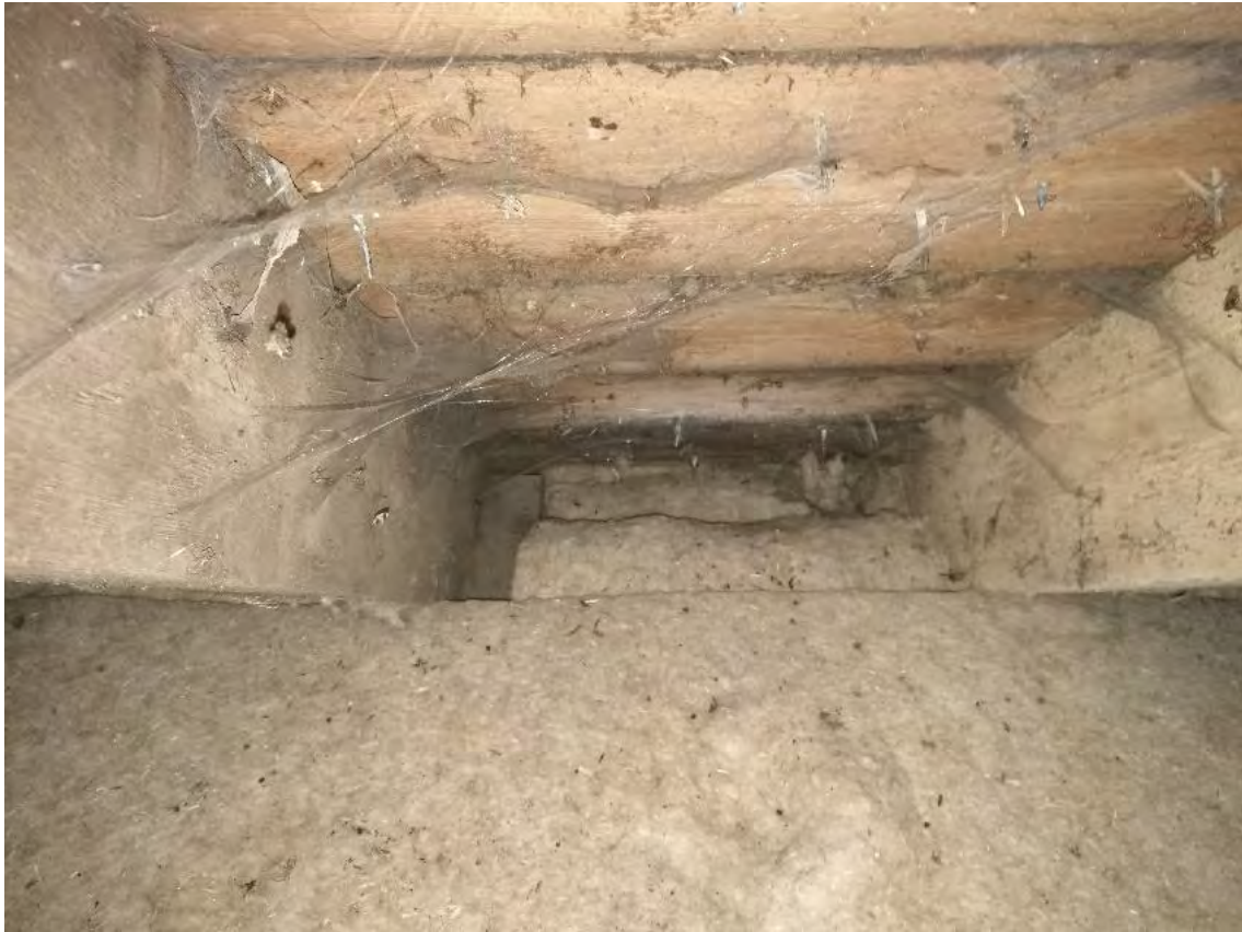
Figure 14: At Scotstarvit Cottage there did not appear to be any air gaps at eaves level to encourage ventilation in the roof space.
