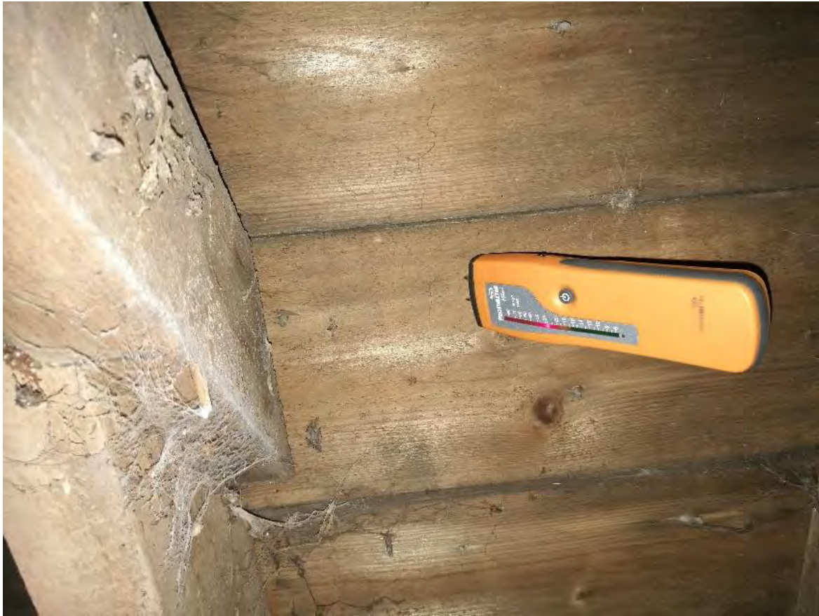
Figure 13: Higher moisture levels recorded on the underside of the sarking boards in the area over the shower room at the Garden Bothy.
