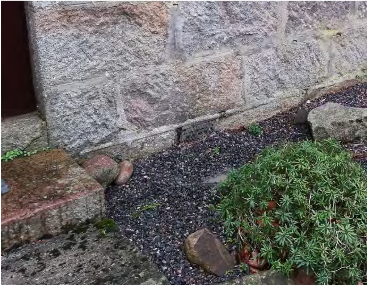
Figure 19: Raised external ground levels and partially blocked underfloor ventilation, as identified at Kirktoon of Coul, can compromise natural airflow into the underfloor space which increases the risk of damp related problems such as condensation and timber decay.
