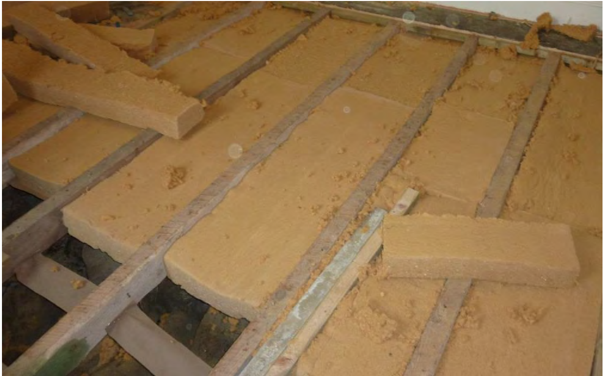
Figure 17: Wood fibre board insulation being installed to a suspended timber floor (Photo courtesy of Historic Environment Scotland).
