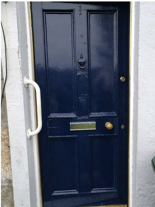
Figure 26: Russell Street, Rothesay. Despite recent re-decoration, the front door is in poor condition, with rot, damaged mouldings and poor preparation. The door remains draughty at the threshold.
