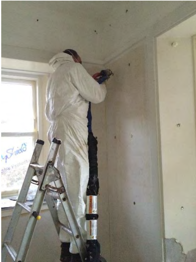
Figure 3: Insulation behind existing wall linings in the form of open cell foam (Icynene) at Annat Road (photo courtesy of Historic Environment Scotland).
