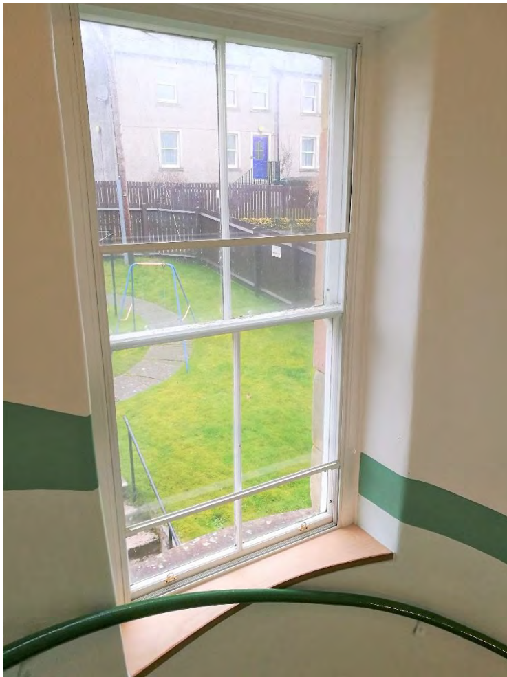
Figure 20: The installation of secondary glazing in Rothesay allowed the original timber sash and case window to be retained but has proved cumbersome to operate.
