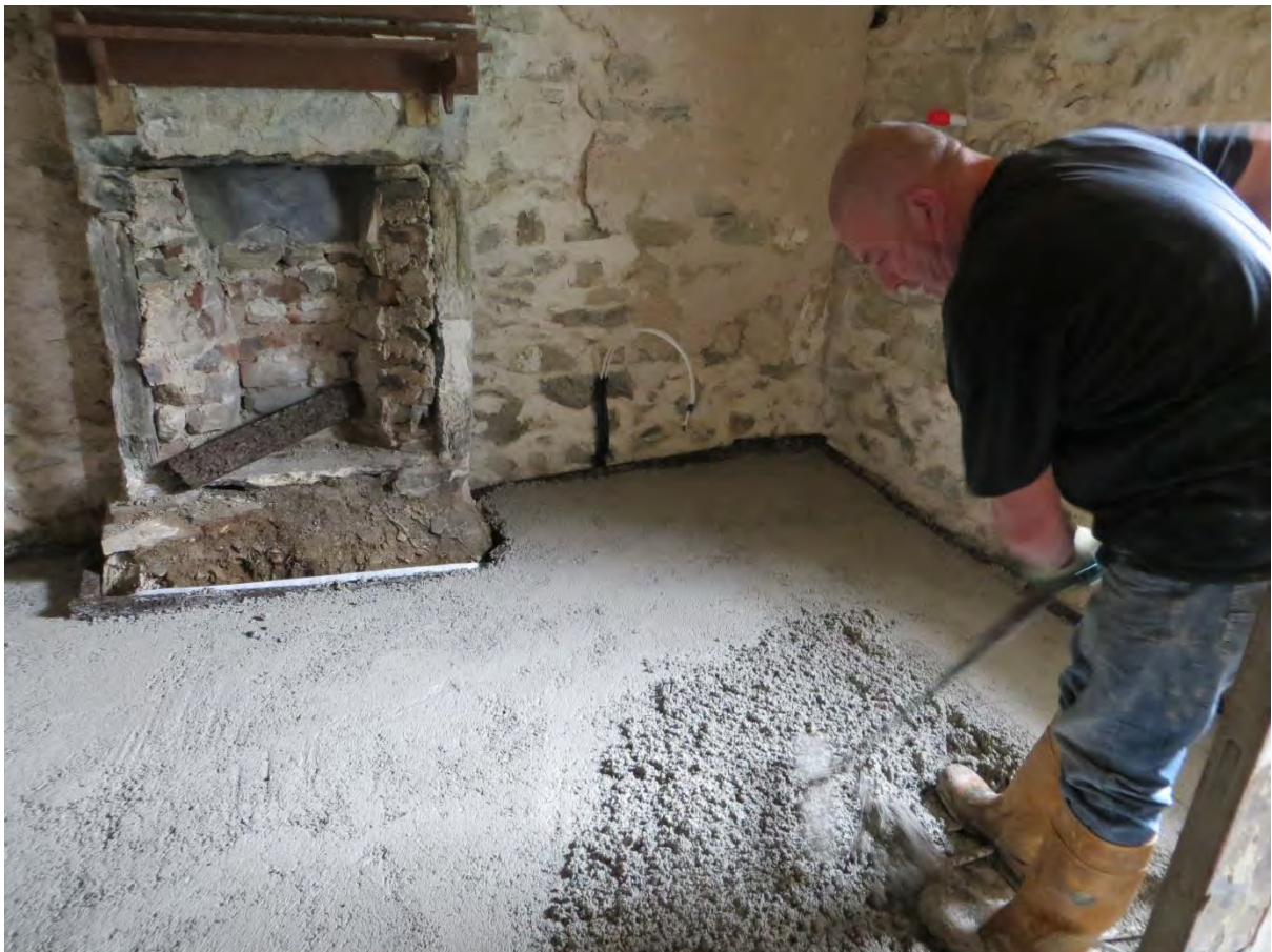
Figure 18: Insulated lime concrete being laid at Downie's Cottage (photo courtesy of Historic Environment Scotland).
