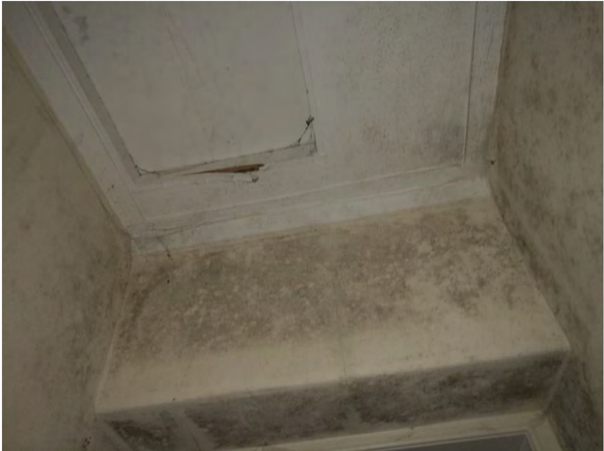
Figure 16: Surface mould in the hallway around the uninsulated loft hatch cover at Wells o' Wearie.
