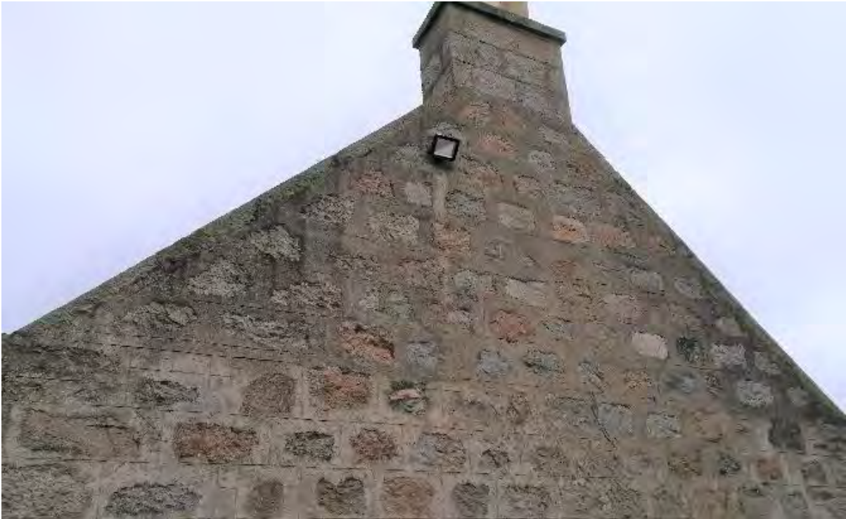
Figure 34: The masonry at Kirkton of Coull. As with Wells o' Wearie, damp masonry is compromising the performance of the new wall insulation. In this case the damp is likely to be exacerbated by the use of cement based pointing.
