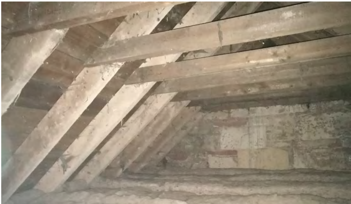
Figure 10: Sheep's wool insulation forming a cold roof at the Garden Bothy in Cumnock.
