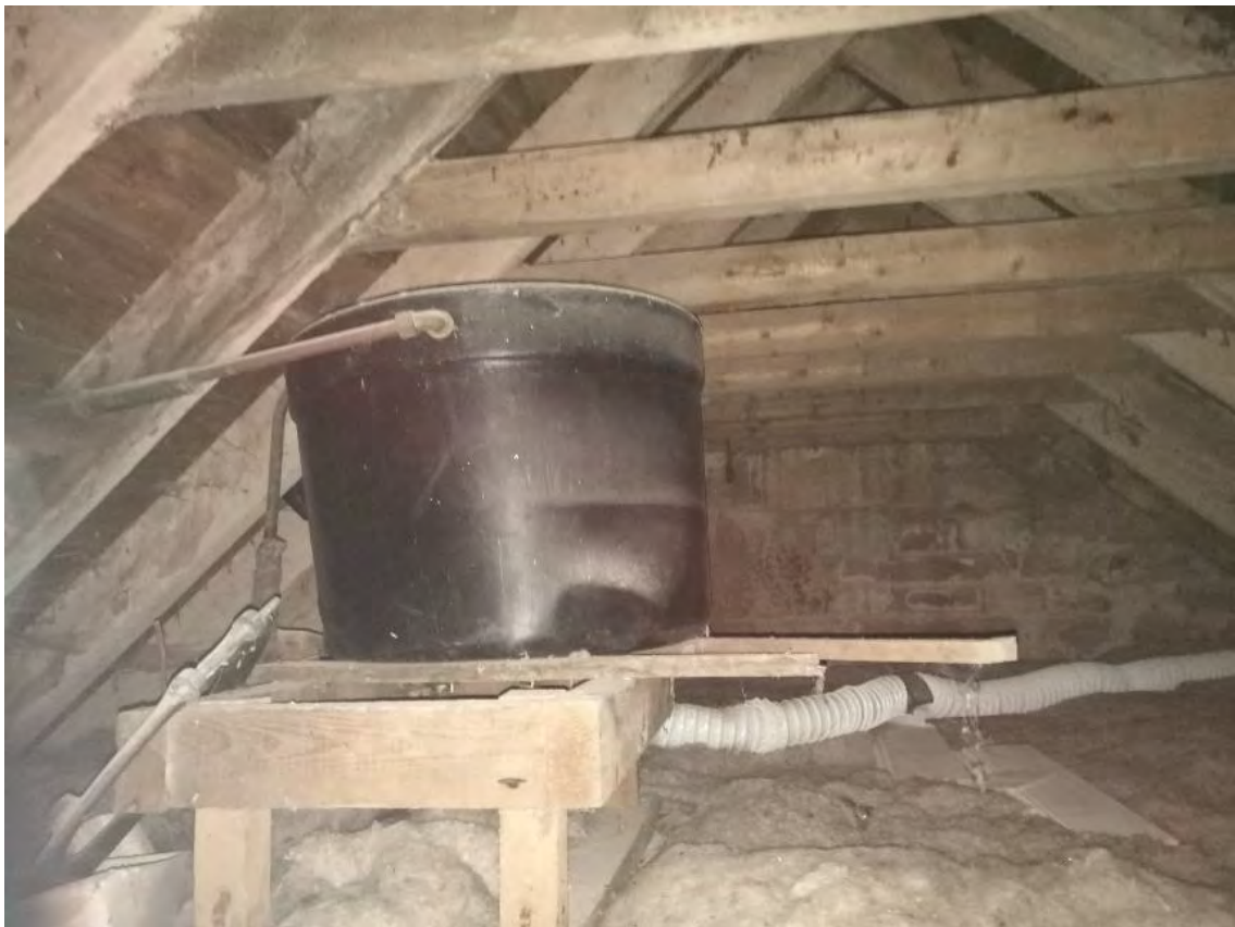
Figure 15: Uninsulated cold water storage tank and associated pipework at the Garden Bothy, which could cause problems if subjected to freezing temperatures.
