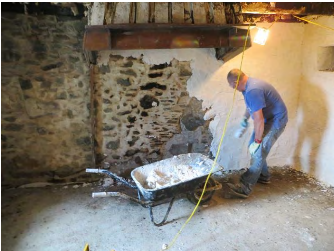
Figure 6: Surface applied insulated lime plaster at Downie's Cottage (photo courtesy of Historic Environment Scotland).
