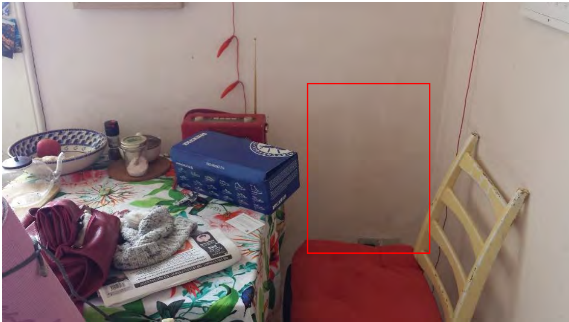
Figure 8: Mould growth (outlined in red) on the wall at Roxburgh Street, Edinburgh.
