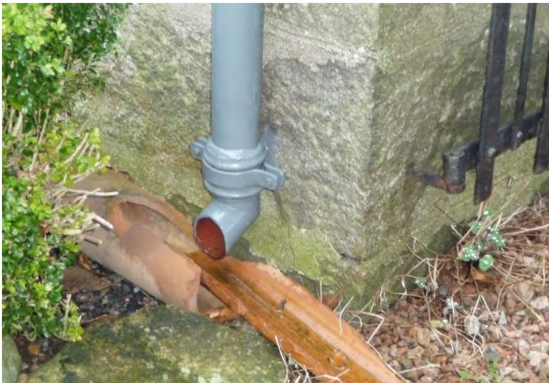
Figure 9: Poor rainwater management in south-east corner of Kirkton of Coull corresponding with area on dampness noted internally in living room.
