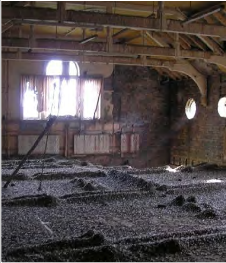
Fig. 1: A roof space with bird droppings.
