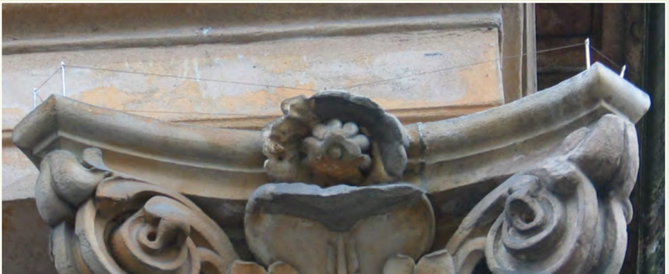
Fig. 6: The top of this column is protected by spring wire attached to vertical supports.
