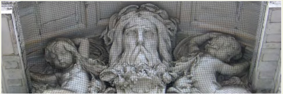
Fig. 3: Netting is used here to protect the detailed carvings over this entrance way.
