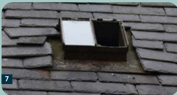
Figure 7. An example of a window needing repair.
