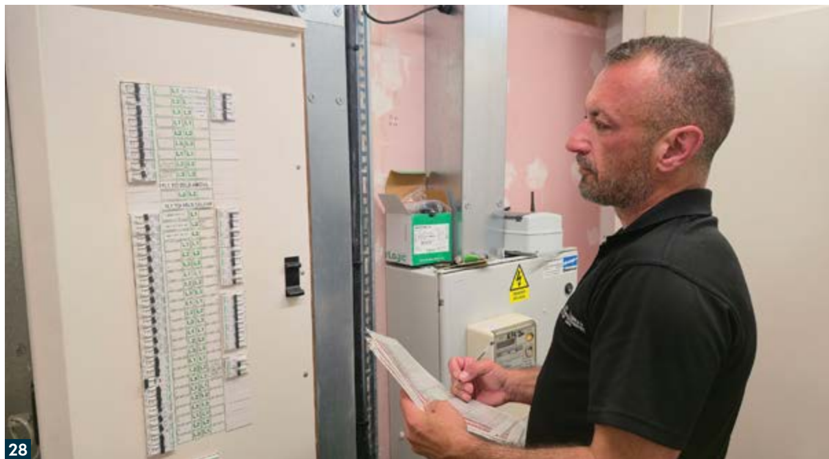
Figure 28. Ensure that all essential building components, such as electrics, are regularly checked by a qualified person.
