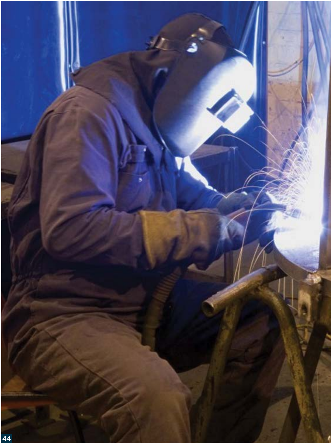
Figure 44. Welding is an example of ‘hot work’ which could pose a fire risk.
