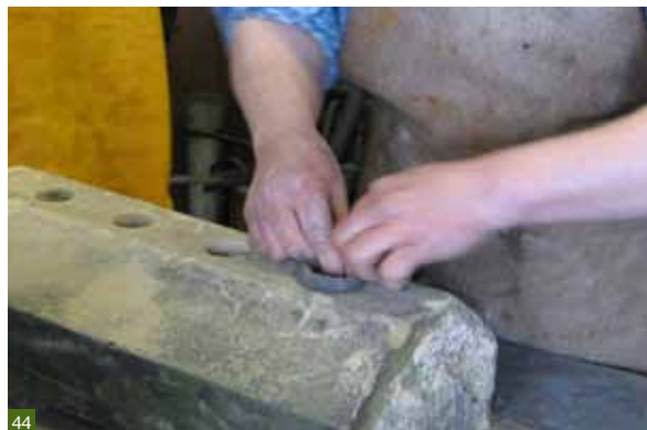
Fig 44 Clay cups are used to prevent molten lead spilling onto surrounding masonry.
