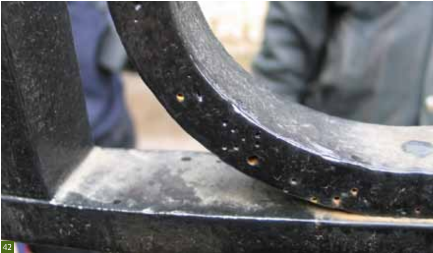
Fig 42 Casting flaws are common in traditional cast ironwork. Care should be taken to fill these before painting to prevent corrosion. Corrosion has begun to develop in the small casting flaws illustrated here.
