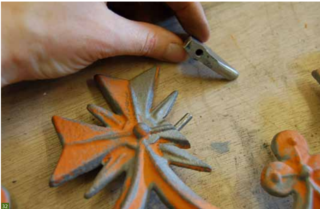
Fig 32 Pinning can be an effective repair where replacement castings need to be joined to original castings.
