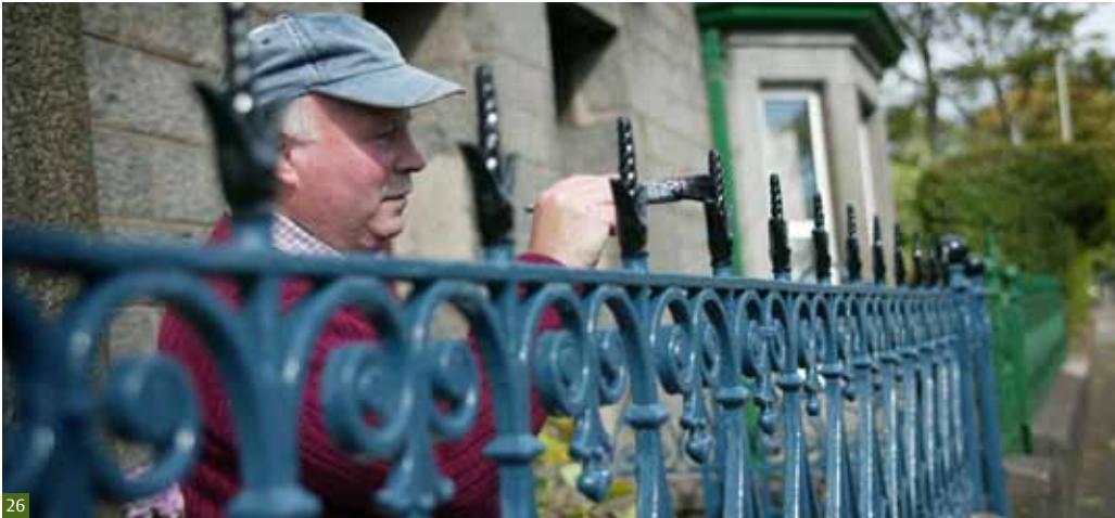
Fig 26 Annual inspections and regular painting will reduce the need for more expensive repairs in the future.
