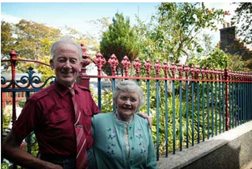
Fig 45 Traditional cast ironwork can enhance the character and appearance of traditional buildings and will survive for a considerable time if well maintained.
