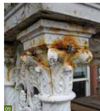
Fig 8 Cracked and flaking paint will trap water and accelerate corrosion.
