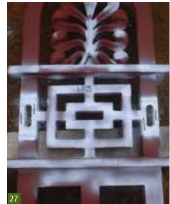
Fig 27 Dye penetration testing can reveal cracks that are not easily visible to the naked eye.
