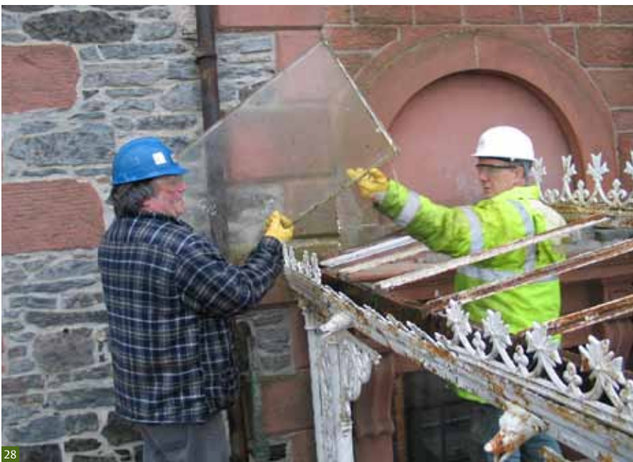
Fig 28 Dismantling in progress. Each element should be tagged according to survey drawings.
