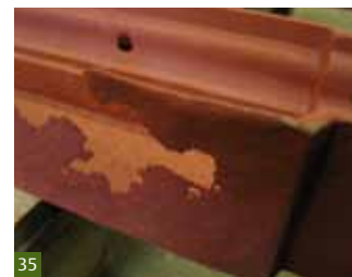
Fig 35 A severe example of corrosion thinning to a thin section of cast iron (in this case a gutter).
