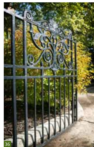
Fig 36 Gates can become difficult to use for a variety of reasons, including raised ground levels and worn components.
