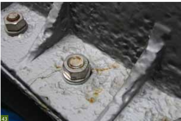
Fig 43 Over-tightening fixings can cause irreversible damage such as cracks and fractures.
