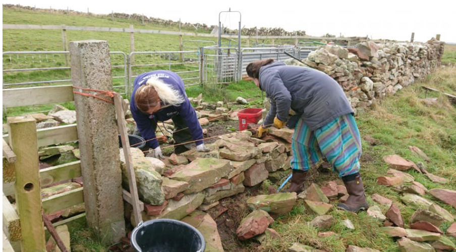
'Cassie' (traditional stone-built sear defence) training course in Papa Westray as part of the North Isles Landscape Partnership Scheme, October 2019.
