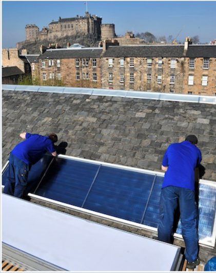
Solar panels being fixed to a roof at Lauriston Place, Edinburgh. Separate guidance on small-scale renewable energy developments is available in Historic Scotland's 'Managing Change in the Historic Environment: Micro-Renewables' guidance note.
