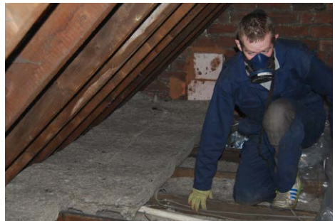
Sheep's wool insulation installed in a loft space which will help to reduce energy demand and improve thermal comfort.
