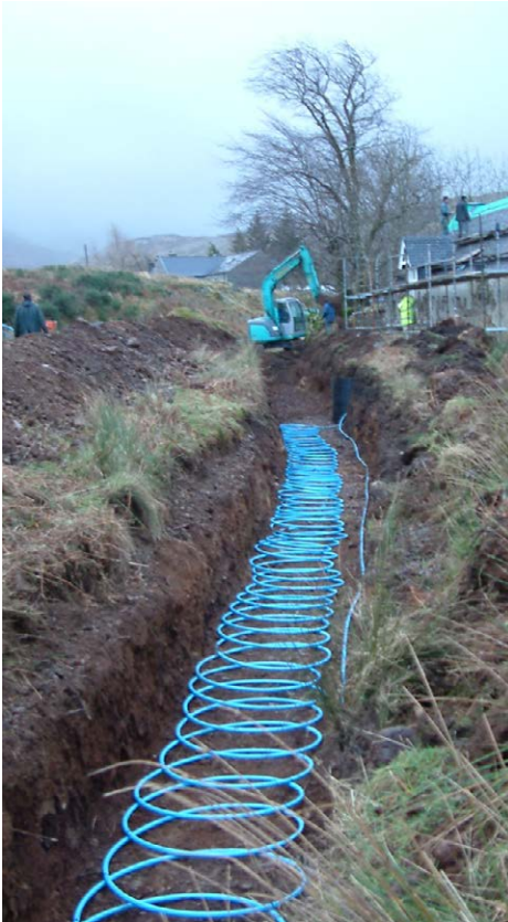
Installation of a ground-source heat pump (GSHP) at Assynt Church, Inchnadamph (Category B-listed). The coils for the system were installed in trenches behind the church. © LDN Architects
