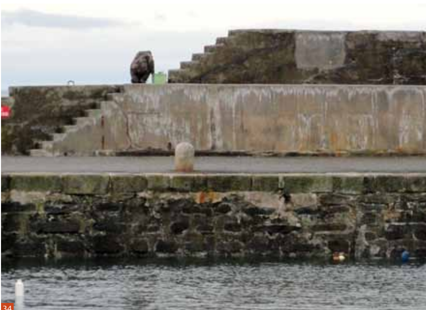
Fig 34 The New Harbour at Portsoy (19th century) showing a poorly matched modern repair to the face of the sea wall.
