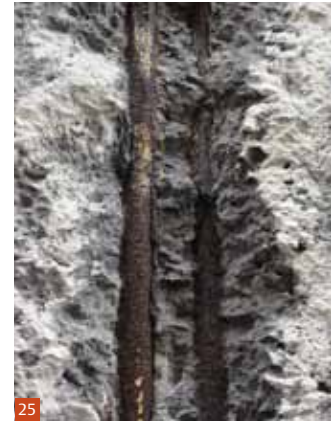
Fig 25 170-2 Hope Street, Glasgow (Lion Chambers) (1905). Due the slender nature of the concrete, limited cover to the reinforcement has allowed carbonation to reach the reinforcement resulting in the serious corrosion.
