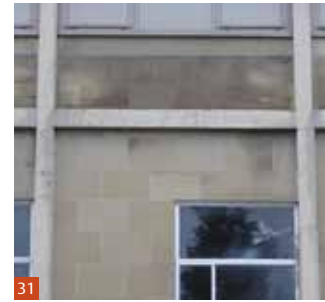
Fig 31 A concrete frame with masonry infill on a 1950s building in Edinburgh. The slender concrete frame provides limited cover to the reinforcement, resulting in its corrosion and cracking of the concrete. © Andrew Wright.
