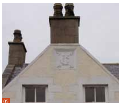
Fig 4 St Aloysius Church, 23, 25 Rose Street, Glasgow (1908-10). A neo-baroque, Jesuit church with concrete roofs and cupolas. The form of concrete construction for the roof is thought to be reinforced.
