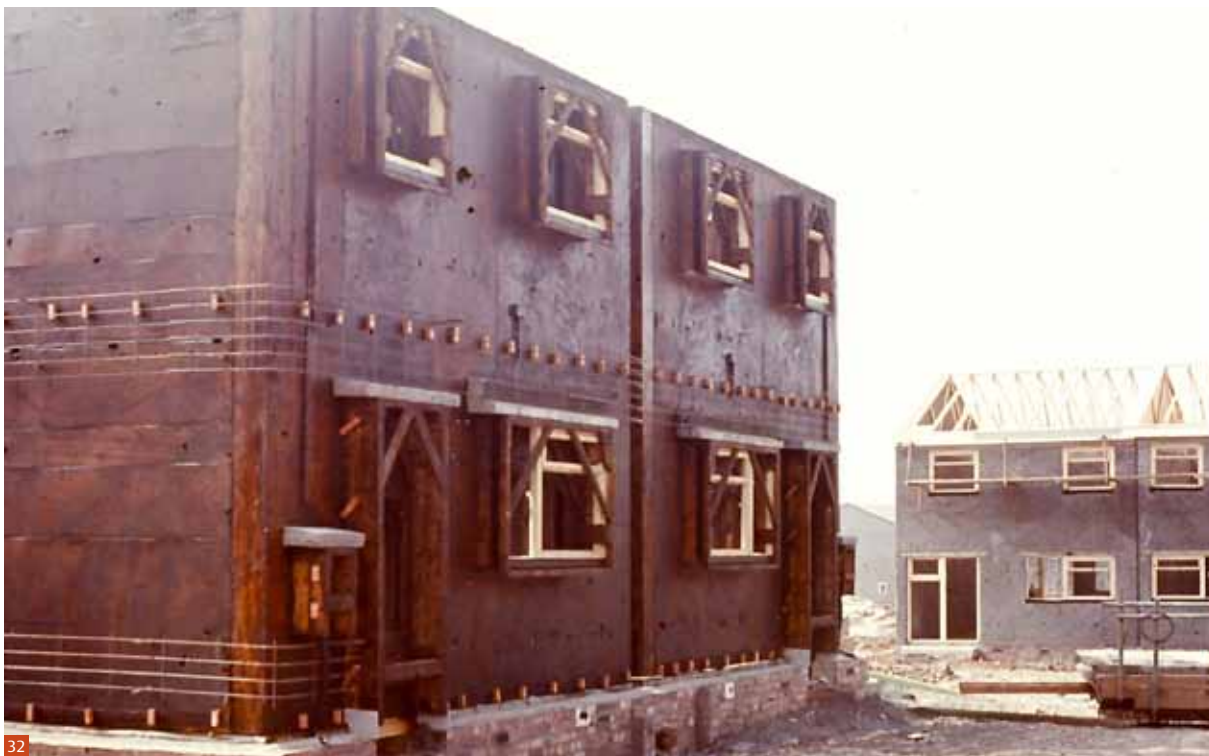
Fig 32 Erection of no fines concrete houses late 1960s. Foreground: two-storey internal shutter ready to receive external shutter and concrete pour.
