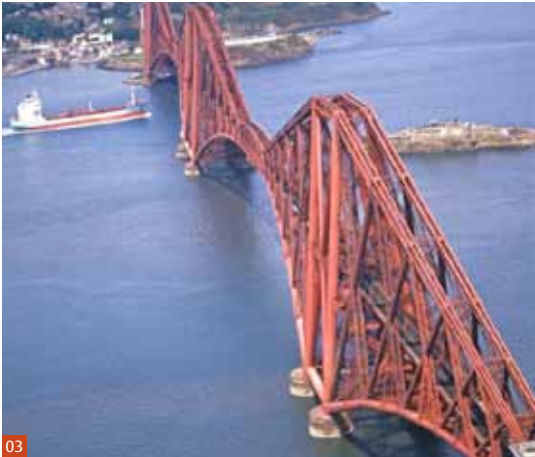
Fig 3 Forth Bridge (1883-90). Britain's first major steel structure is supported upon concrete and masonry piers. © Historic Scotland
