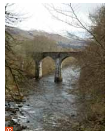
Fig 2 Killin rail viaduct over the River Dochart (1885-86) is the second oldest mass concrete viaduct in Britain after the Falls of Cruachan. © Historic Scotland
