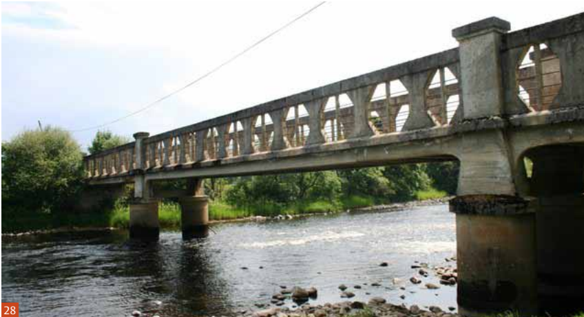
Fig 28 Advie Bridge over the River Spey, Cromdale, Highland (1921-22). Three-span concrete bridge with reinforced concrete trusses on paired concrete piers.
